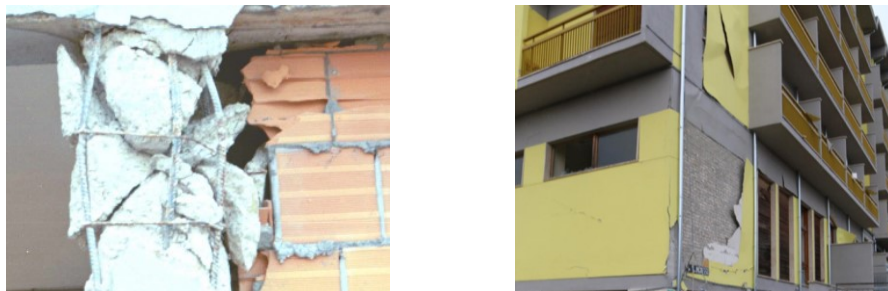
Figure 1. (left) Shear failure of column (Bonafro, Molise 2002; Magenes and Pampanin [2004]); (right) damage to masonry infill panels and external thermal insulation after the Amatrice 2016 earthquake [Santarsiero et al. , 2016].
