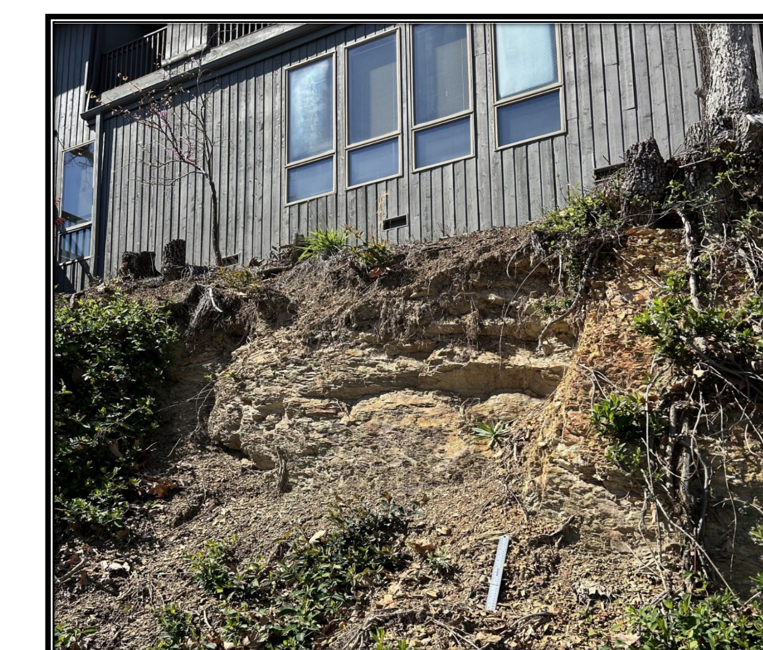
Figure 6: A steep slope showing outcrop of Sevier Shale, this area has had slope failures as recent as 2022.
