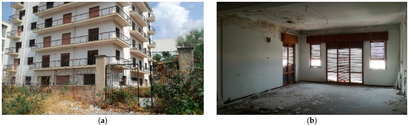
Figure 4. State of the case study RC building: (a) external view and (b) example of internal view.
