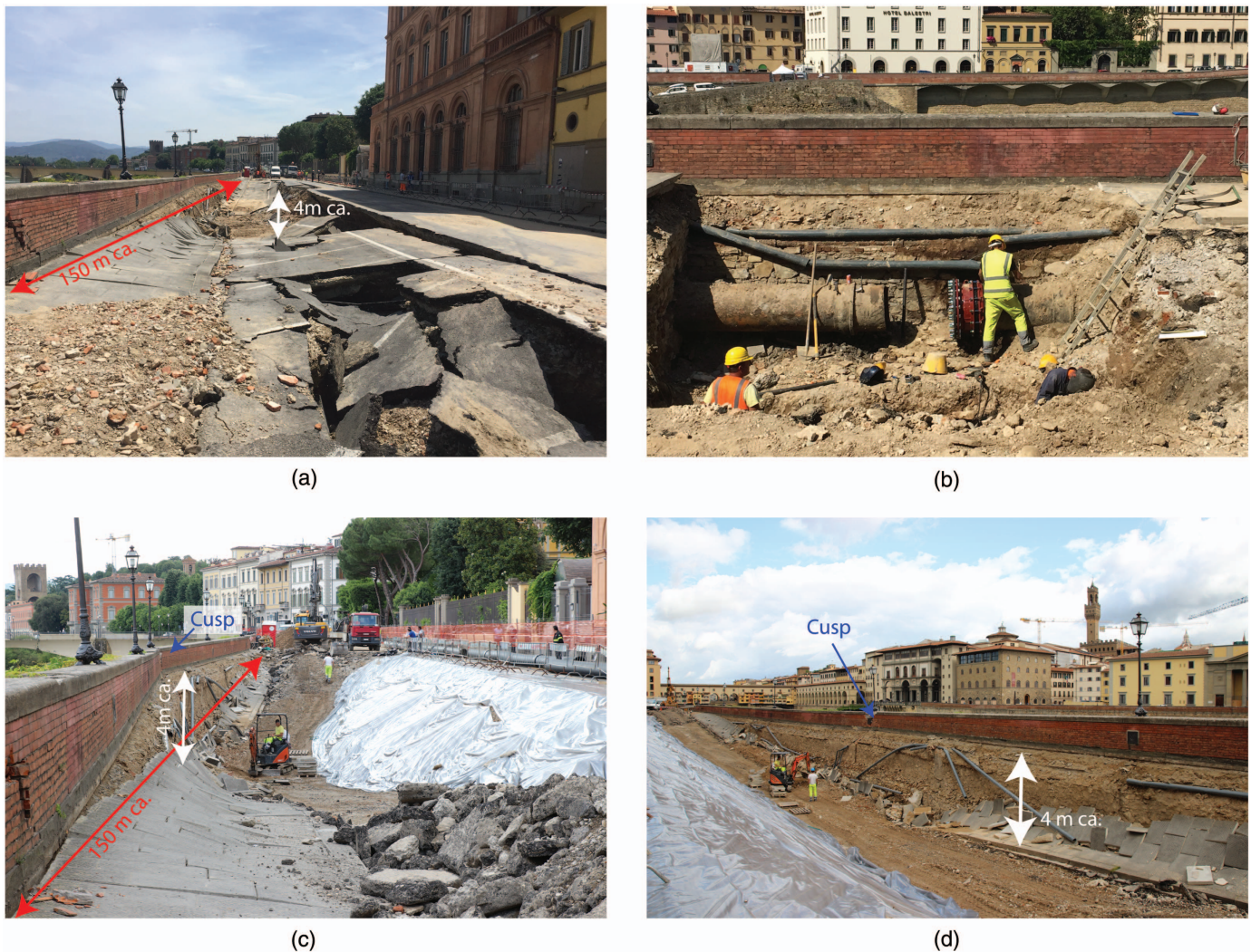
Fig. 4. (Color) Photos show (a) roadway and moved retaining wall immediately after removal of vehicles stuck inside landslide; (b) repair of big pipeline affected from catastrophic failure; and (c and d) construction site setup stage (notice large tarps for temporary protection). (Images by M. Nocentini.)
