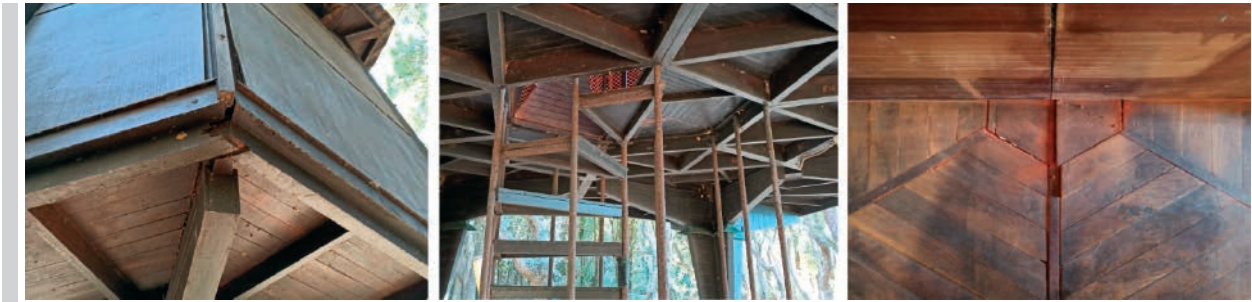
Figure 3. Loosening of slab joint, stair's structure corrosion, flooring and wall cladding deformations [source: photo by S. Landi]
