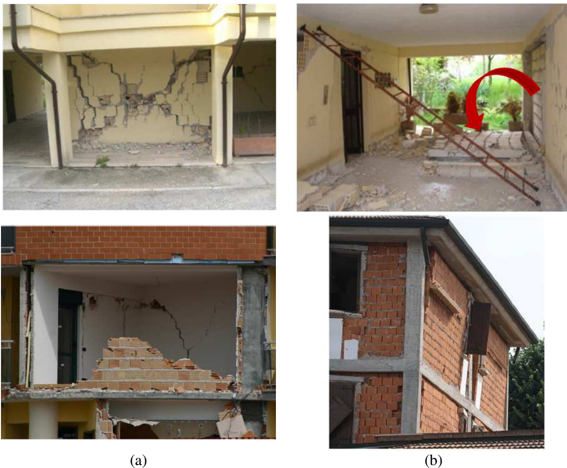
Figure 1 Infill masonry walls earthquake damage in L'Aquila: a) in-plane diagonal cracking, b) out-of-plane collapse (Furtado et al. (2016), Marinković (2019))
