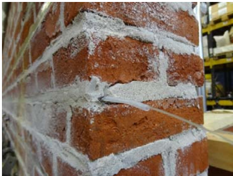
Figure 1: Ends of the optical fibre (pig tails) at the entrance point in the mortar joint
