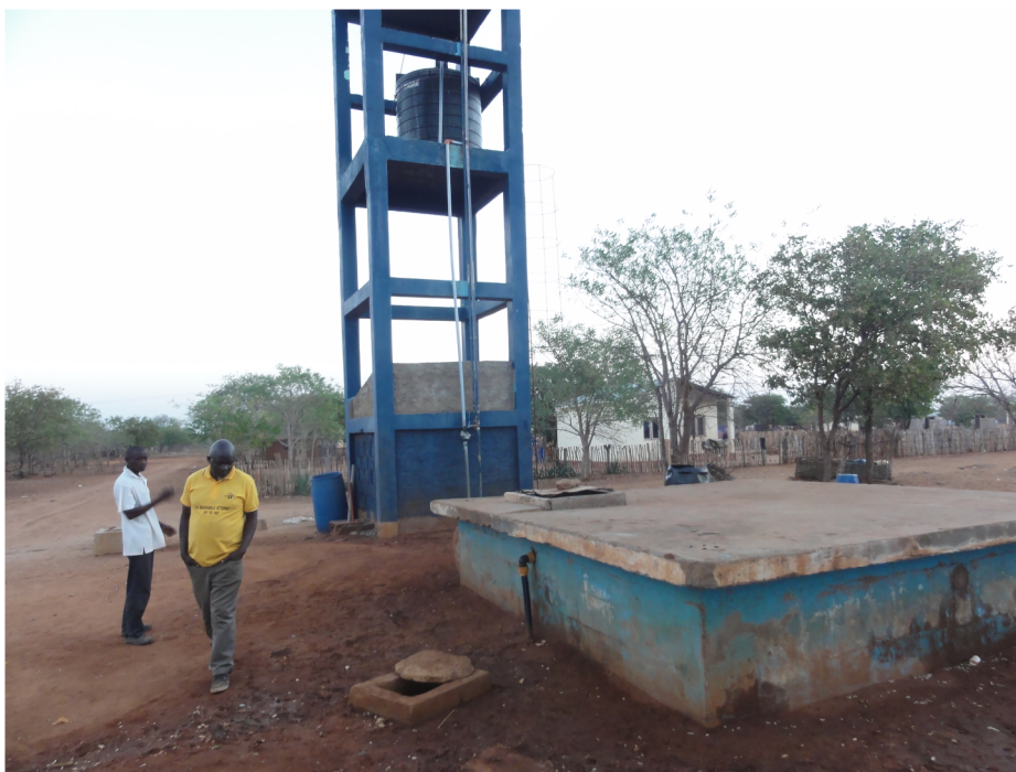
Figure 2. Broken water tank and pump system in Makavene-Banga.
