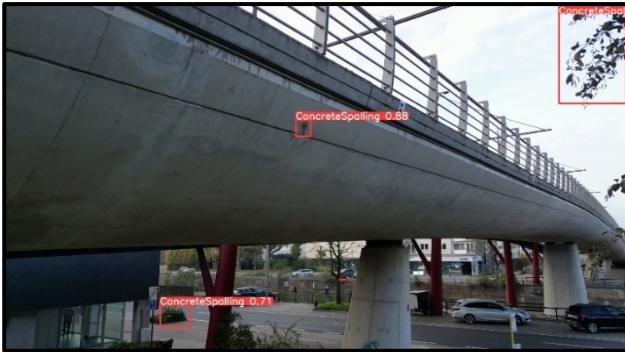
Figure 2: Prediction results with bounding boxes (red) of the YOLOv8 concrete spalling model. The result includes one true positive and two false positive predictions.
