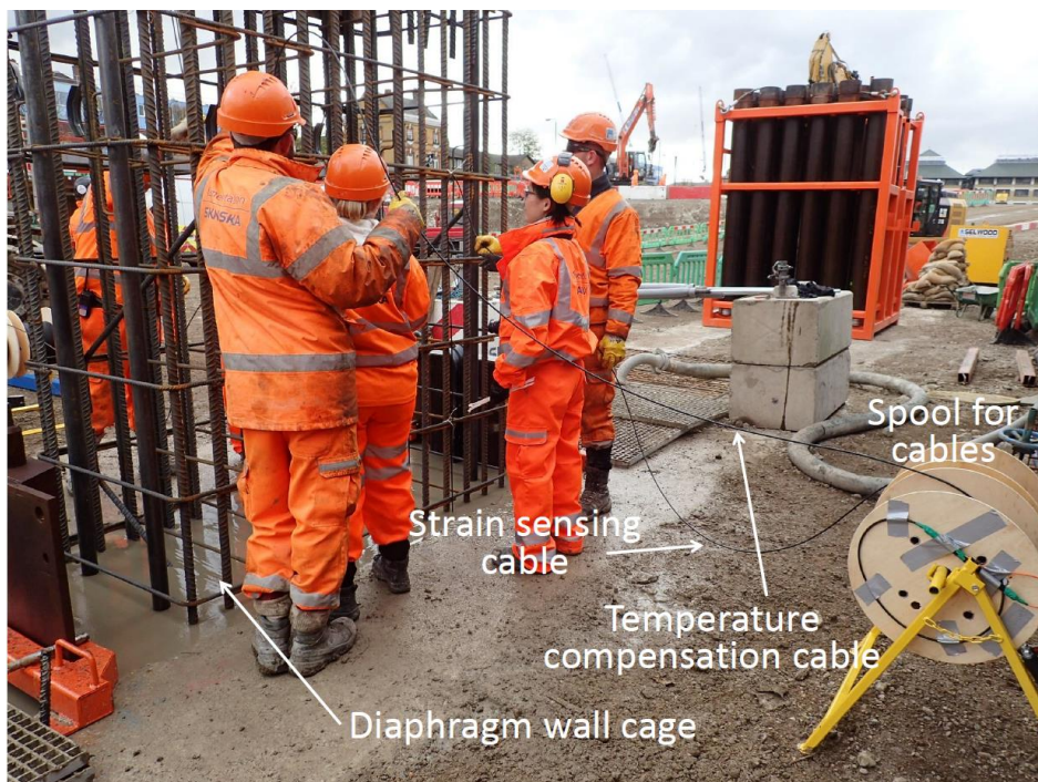
Figure 2.14: Laying cables to measure the temperature and strain at ground level (reprint from (Li, Soga, & Kechavarzi, 2018))
