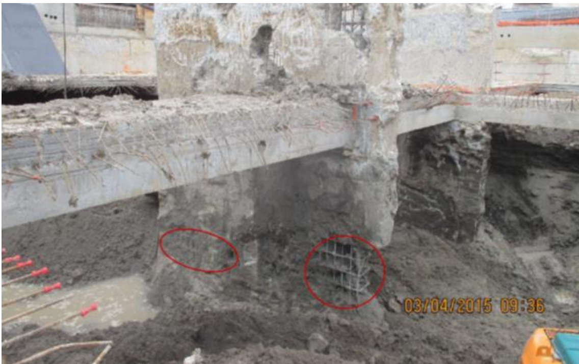
Figure 2.22: Inclusion defects in diaphragm wall (reprint from (Hill & Thorp, 2021)).
