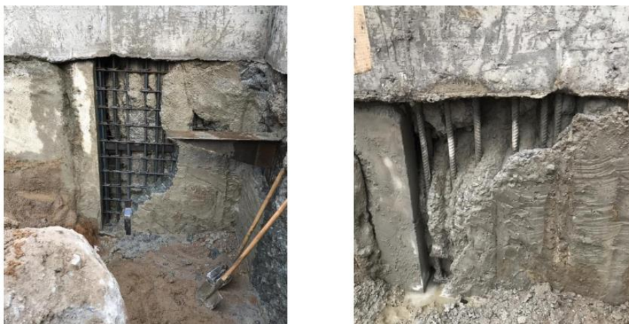
Figure 2.19: Imperfections due to the low flowability of concrete (reprint from (Mironov, Osokin, Loseva, & Kuzhelev, 2020)).
