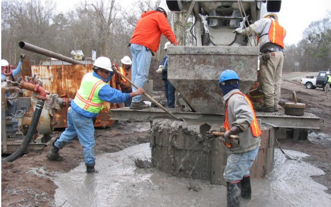
Figure 2.23: Replacing contaminated concrete at the top of a deep foundation using tremie method (reprint from (Brown, Turner, Castelli, & Loehr, 2018)) Copyright © 2018 Dan Brown and Associates, PC
