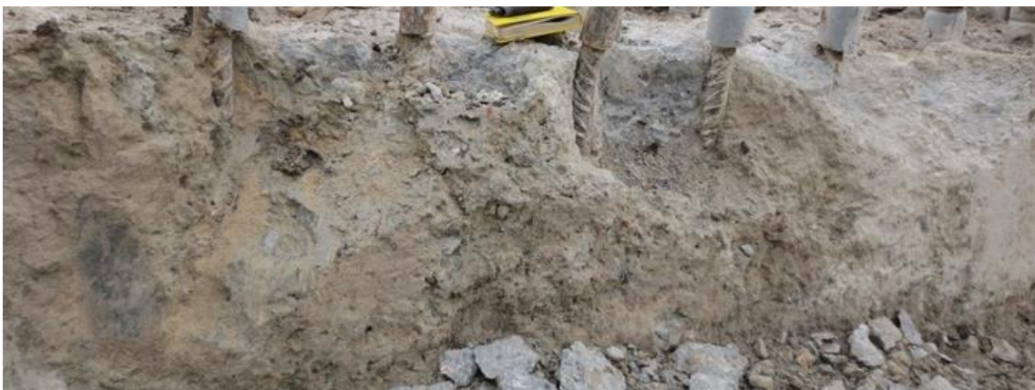
Figure 2.24: Contaminated concrete atop of a diaphragm wall (reprint from (Hill & Thorp, 2021)).
