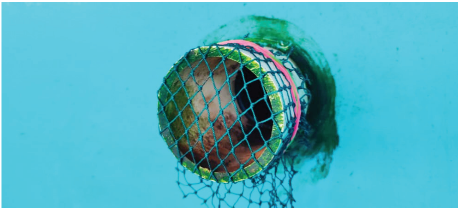
Figure 6. Tank top drain.
