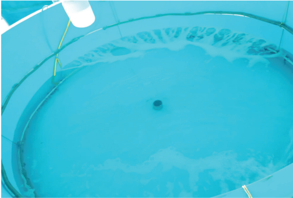
Figure 8. Aeration pipe line in RAS tank
