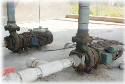
2 HP Motor pumps
