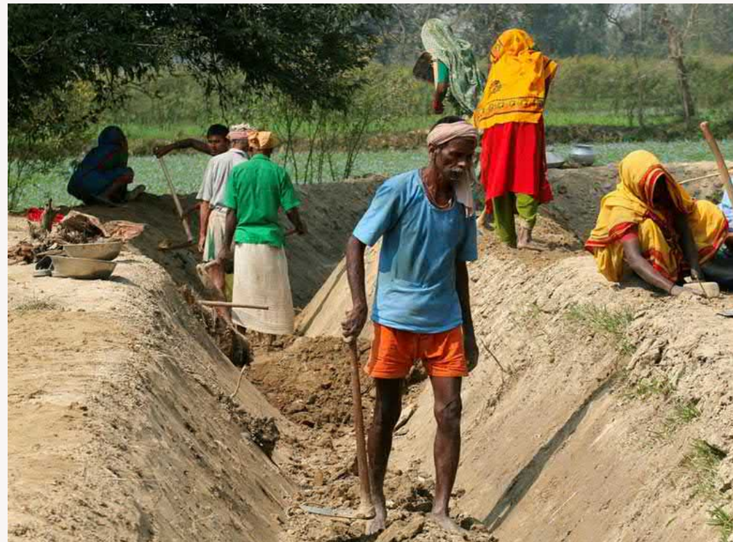
Nepalese workers are building an irrigation ditch in Dhanusha District on 18 February 2009. © ILO
