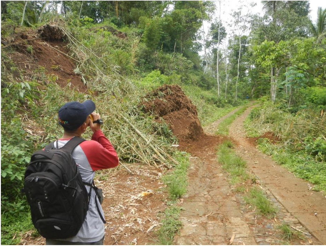
Figure 4.5 Small landslide in Bompon watershed threatening the road infrastructure. Despite the thick vegetation on the surface, the landslide still occurs in several areas in the Bompon watershed.
