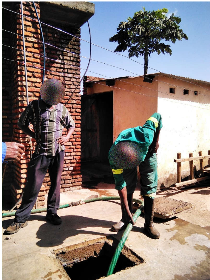
Figure 18 Septic tank emptier. Image: Author's Own
