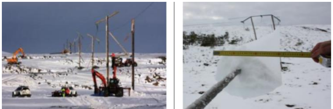
Figure 1.6 A broken 132 kV overhead transmission line (left) and ice accretion on a 132 kV tower with an ice thickness of 20 to 30 cm (right) [1]
