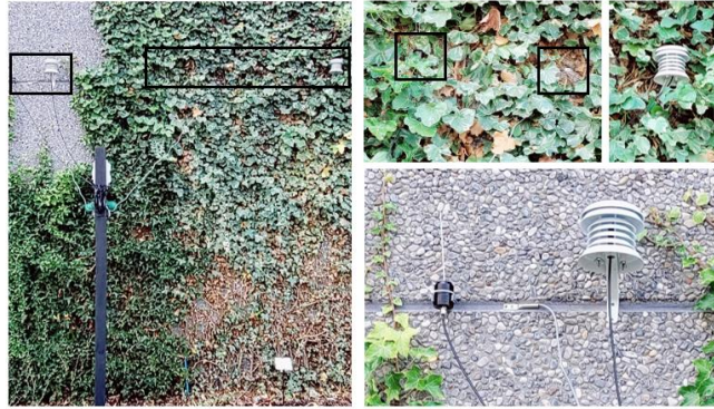
Figure 1. Set-up of monitoring devices on the wall of the case study in Destelbergen with a set-up on the bare wall and a set-up in the vertical greening ( Hedera Helix 'Glacier' ).
