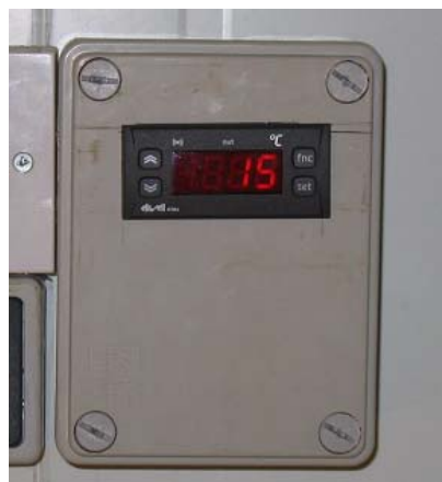
Photo 3.1h: Chilled ceiling temperature controller
