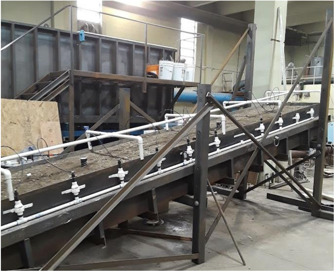
Fig. 10. Watering system pipe network.
