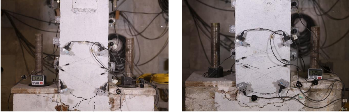
Figure 7-6. Final state of repaired columns after testing. S-20-Rep (left) and S-15-Rep (Right).
