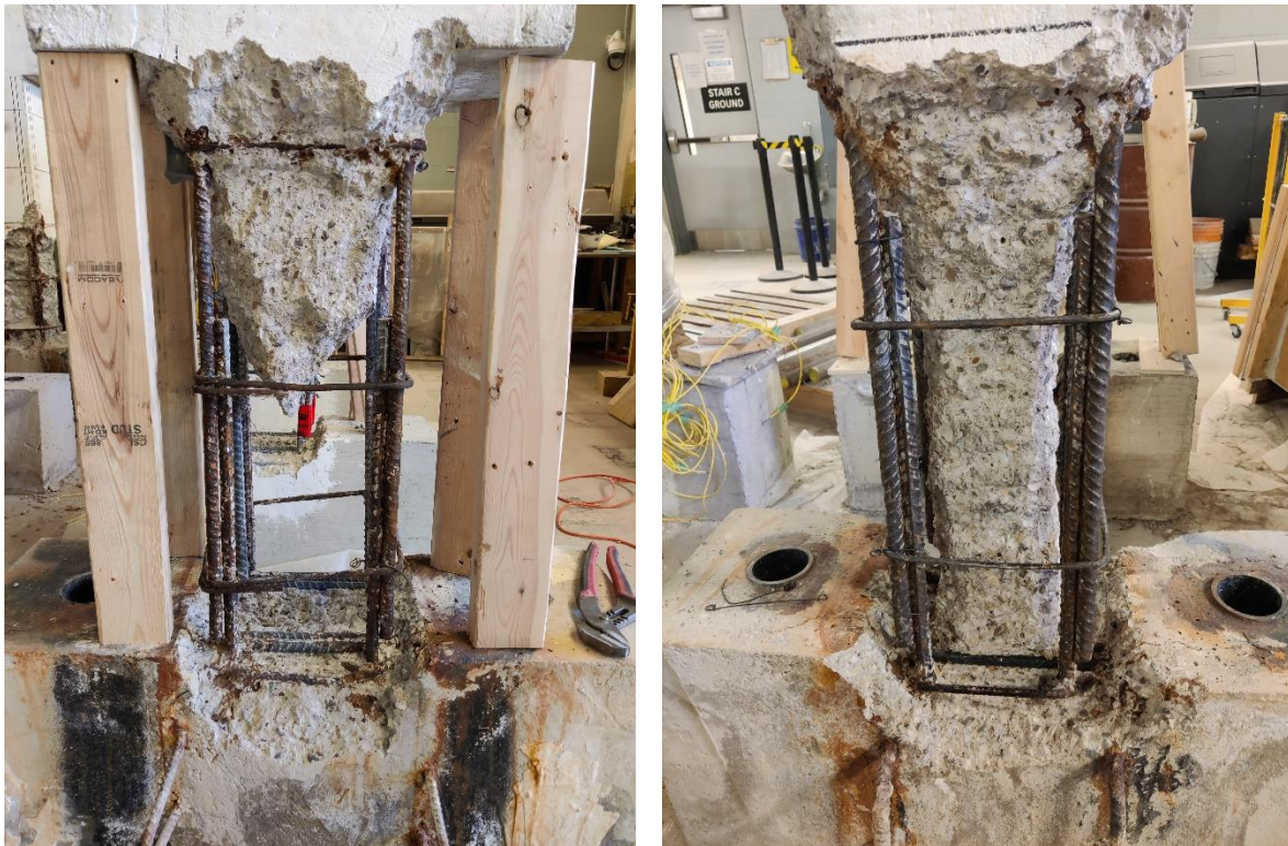
Figure 6-24. Sample of the state of the columns after concrete removal during the repair/strengthening process
