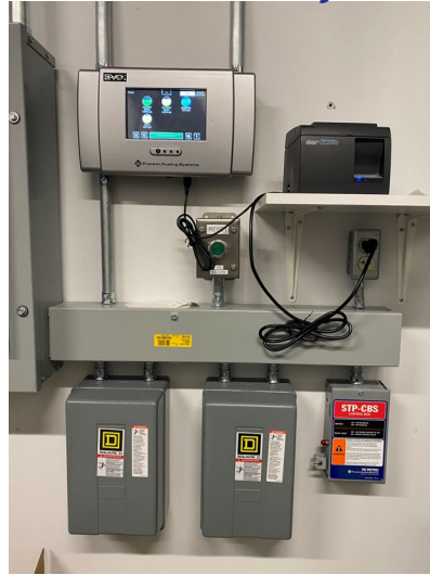
Fuel Depot Usage Monitoring System
