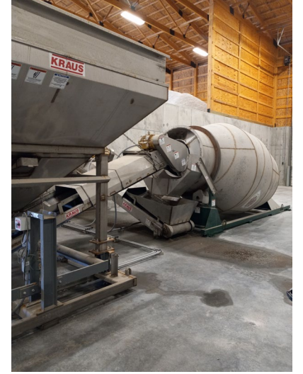
Road Salt & Sand Mixing
