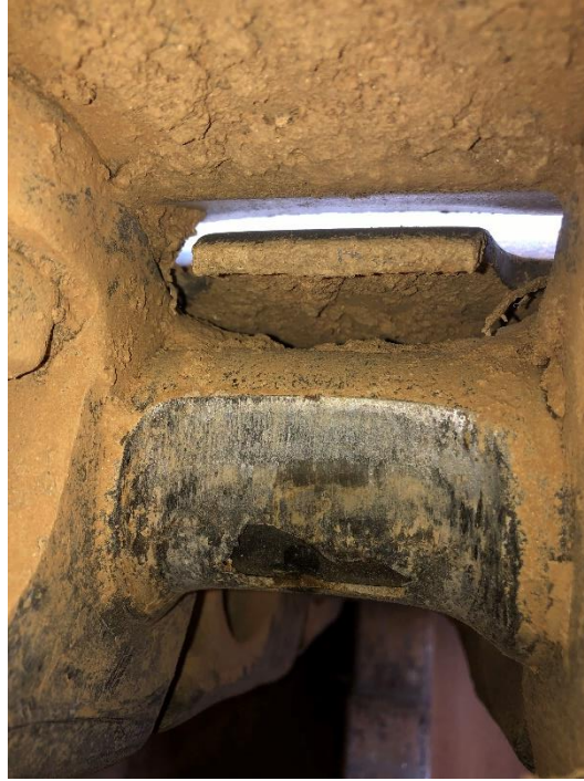
Figure 7. Failed Track Bushing Due to Missed Maintenance
