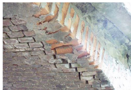
Fig. 2: Opening and falling mortar from joints in a brick vault.
