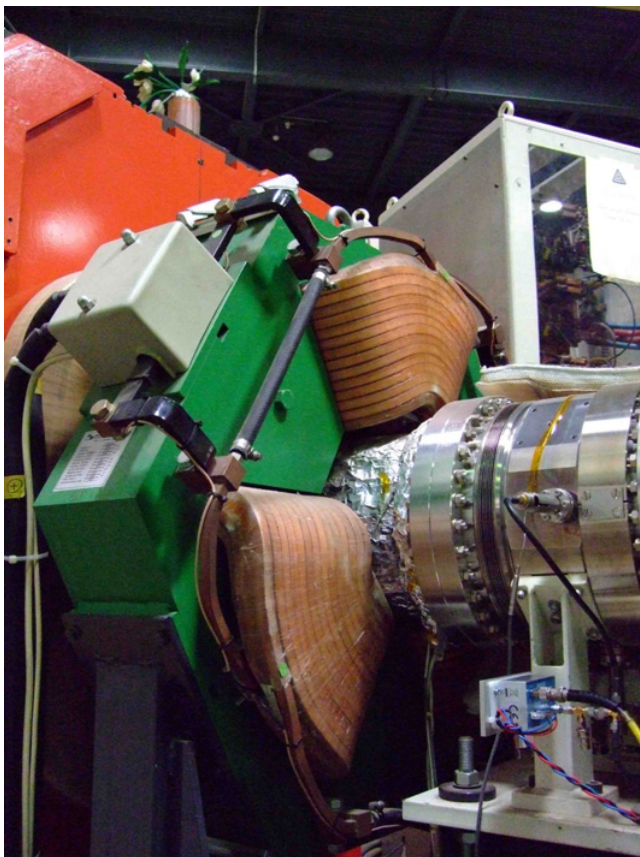
Fig. 32. TSR sextupole magnet. In the front of the sextupole magnet a capacitive pick up to measure the closed orbit of the ion beam is recognizable.
