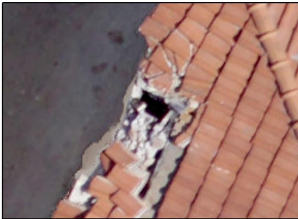
Figure 9. Part of the 25 th July 2017 orthophoto map at a scale of 1:40 which clearly shows damages of grade 2 on the top of the buildings, e.g. collapse of a chimney.
