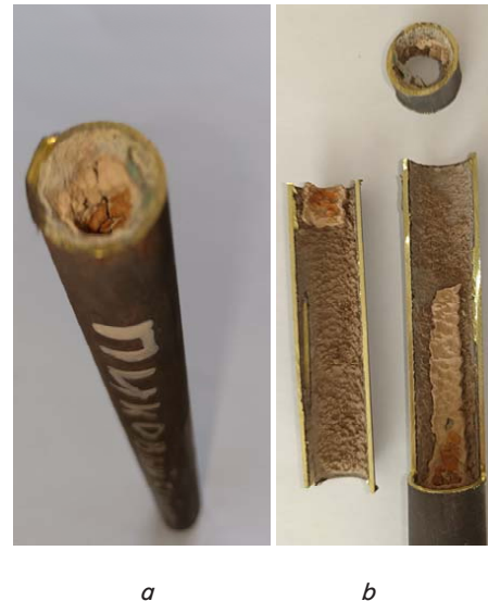
Fig. 3. Peak heat exchanger: a – photo of the scale formed inside the peak boiler; b – images of the peak boiler
