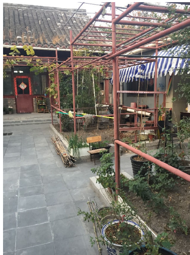
Figure 7-3 the column under unprofessional maintenance and windows in use (above);
