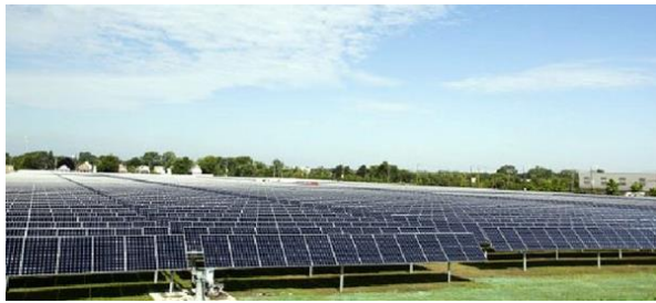
Figure 6.1. SunPower PV panels mounted in single-axis tracker systems in Exelon City Solar (Source: SolarServer)
