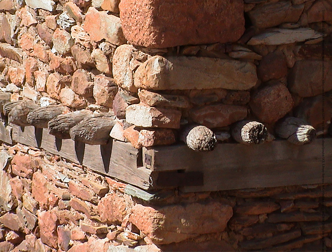
Figure 4. Monkey-head technique, Asmara: Africa's Modernist City. Nomination Dossier for UNESCO World Heritage Listing, Asmara Heritage Project., 2016. [Color figure can be viewed at wileyonlinelibrary.com ]
