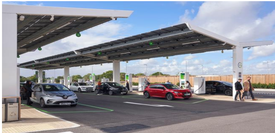
Figure 5.2. Gridserve Electric Forecourt®, Essex, UK. Source: Gridserve™ 2022
