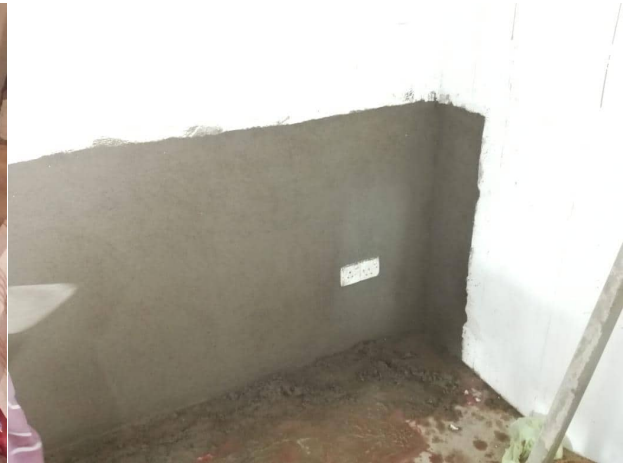
d) final retrofit wall; note that the retrofit looks no different than the existing plastered wall shown in part a)
