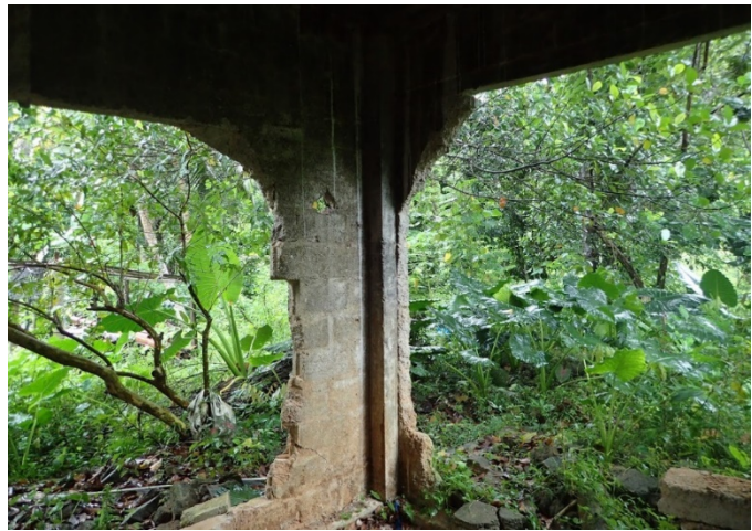
b) complete collapse of single leaf infill walls
