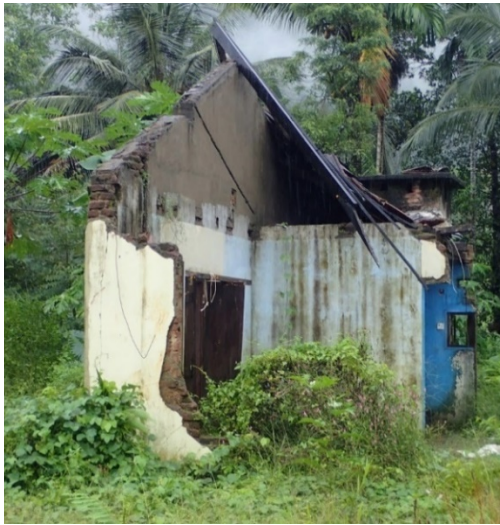
a) complete collapse of load bearing URM
