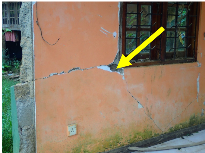
d) failed external walls and flexural cracks
