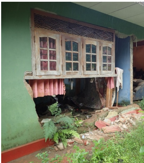
c) flexural failure parallel to bed joint (note the elevated window height)
