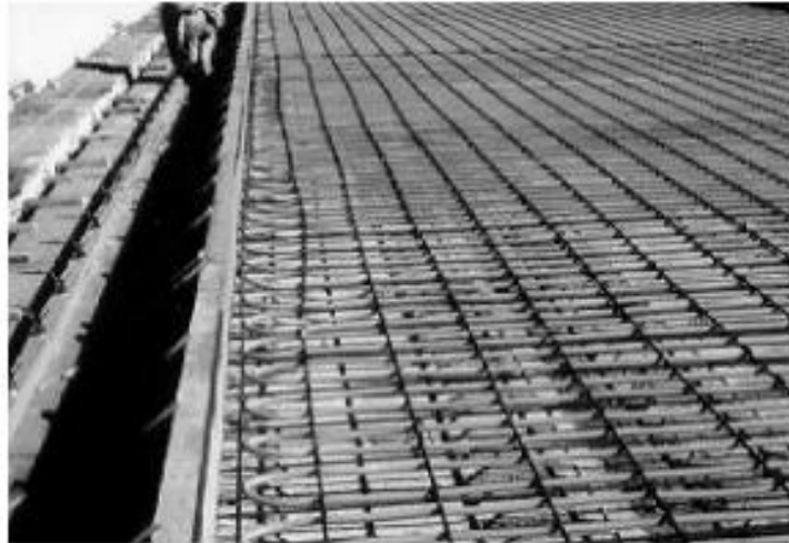
Figure 15. Amarillo, TX geothermal heating system construction: heating hoses in place ready for concrete pour
