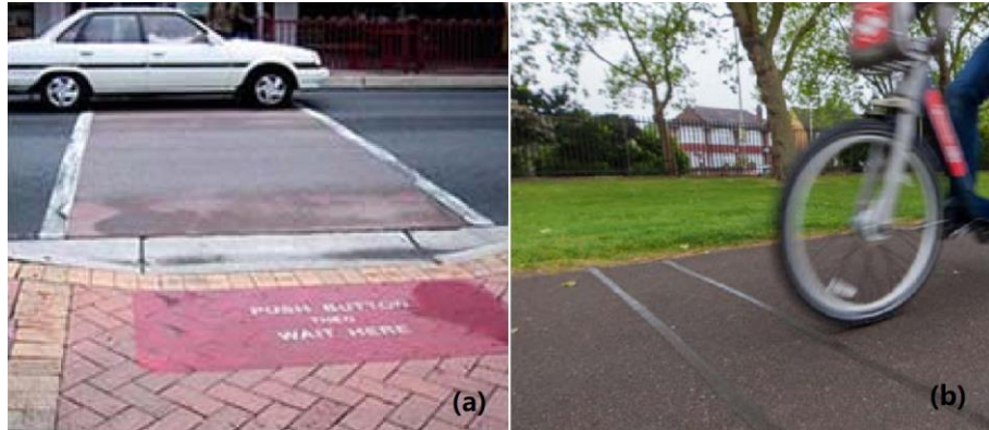
Figure 33. (a) piezoelectric mat for detecting pedestrian; (b) piezoelectric cable for detecting bicycles
