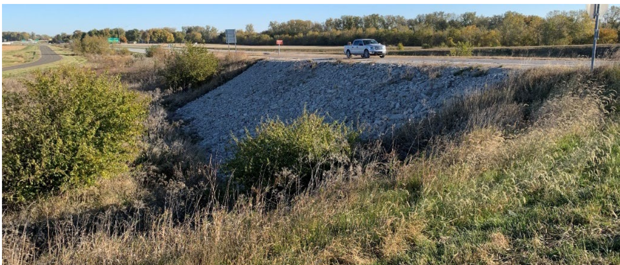
Figure 3-6: Example of a successfully mitigated soil slope failure inventoried in the GAM application.
