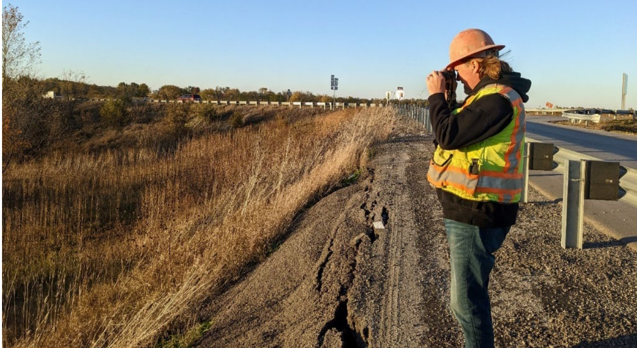
Figure 3-5: Soil slope failure assessed and inventoried in the GAM program. Note ground cracks immediately left of the inspecting geologist.
