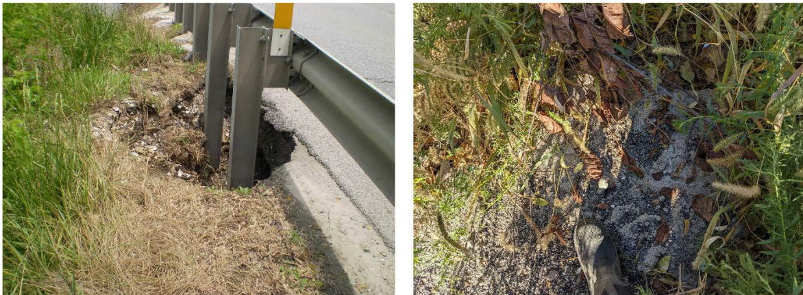
Figure 3-7: Pair of photographs of a sinkhole near the Hwy 24 bridge at Quincy showing 2010 conditions (left) and post-mitigation conditions in 2022 (right).
