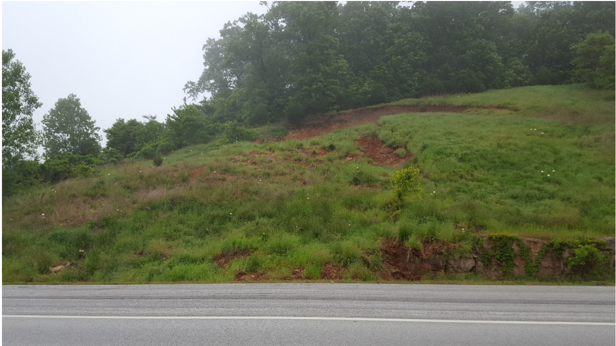
Figure 4: Reflective monitoring stations from previous research on the Ozark Mountain Highroad Slide in May 2020.
