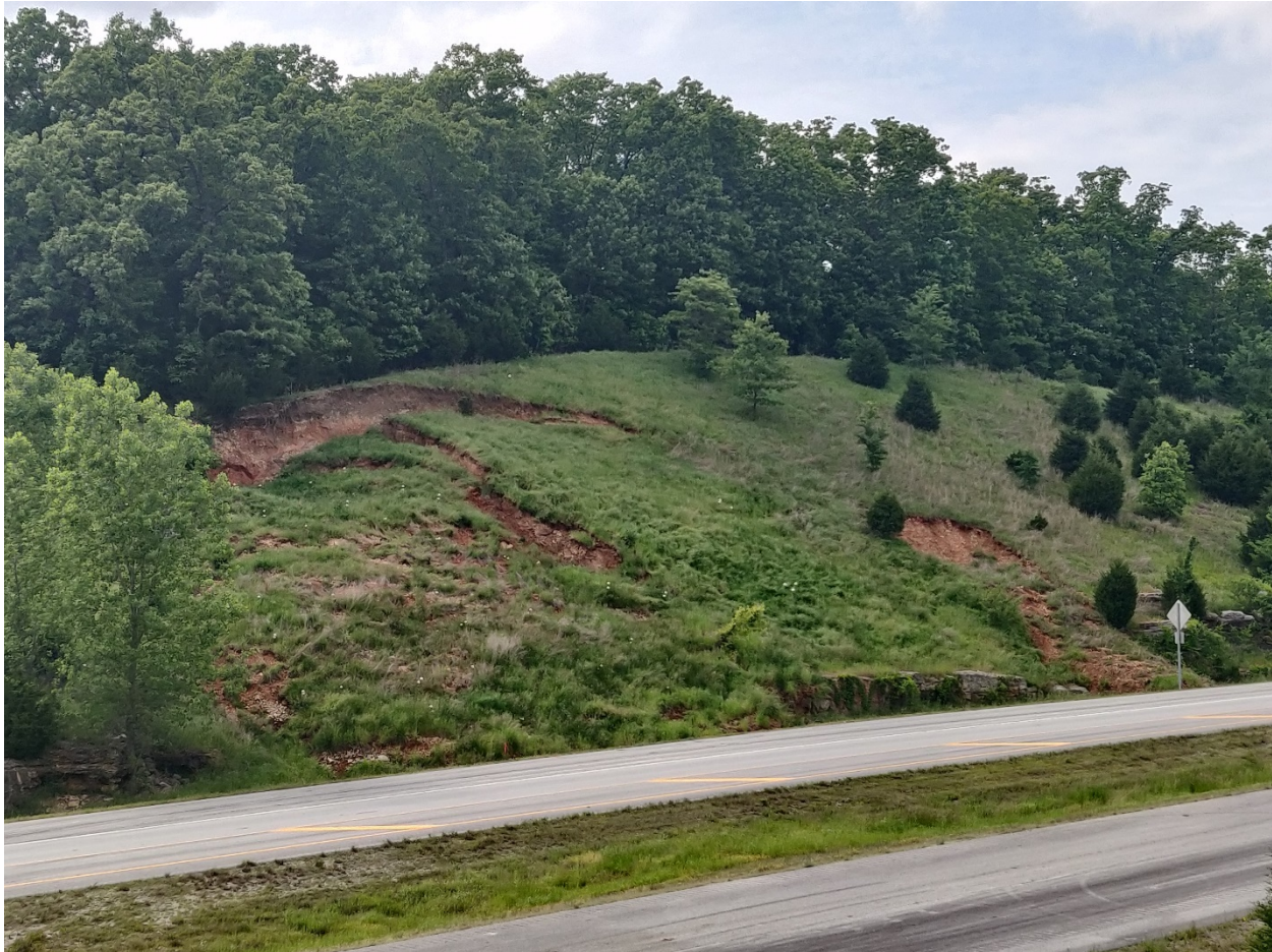
Figure 8: View of cut slope landslide complex taken from the Route 76 overpass May 2020.
