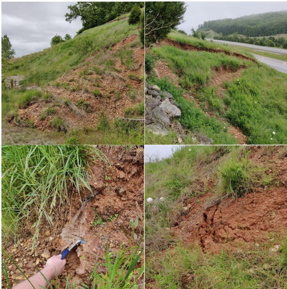
Figure 9: Slide features from May 2020. Clockwise from left, toe deposit in the roadway ditch, nested scarps at the head of the slide, an internal toe in the slide mass, and water seeping from the recently mobilized slide debris.
