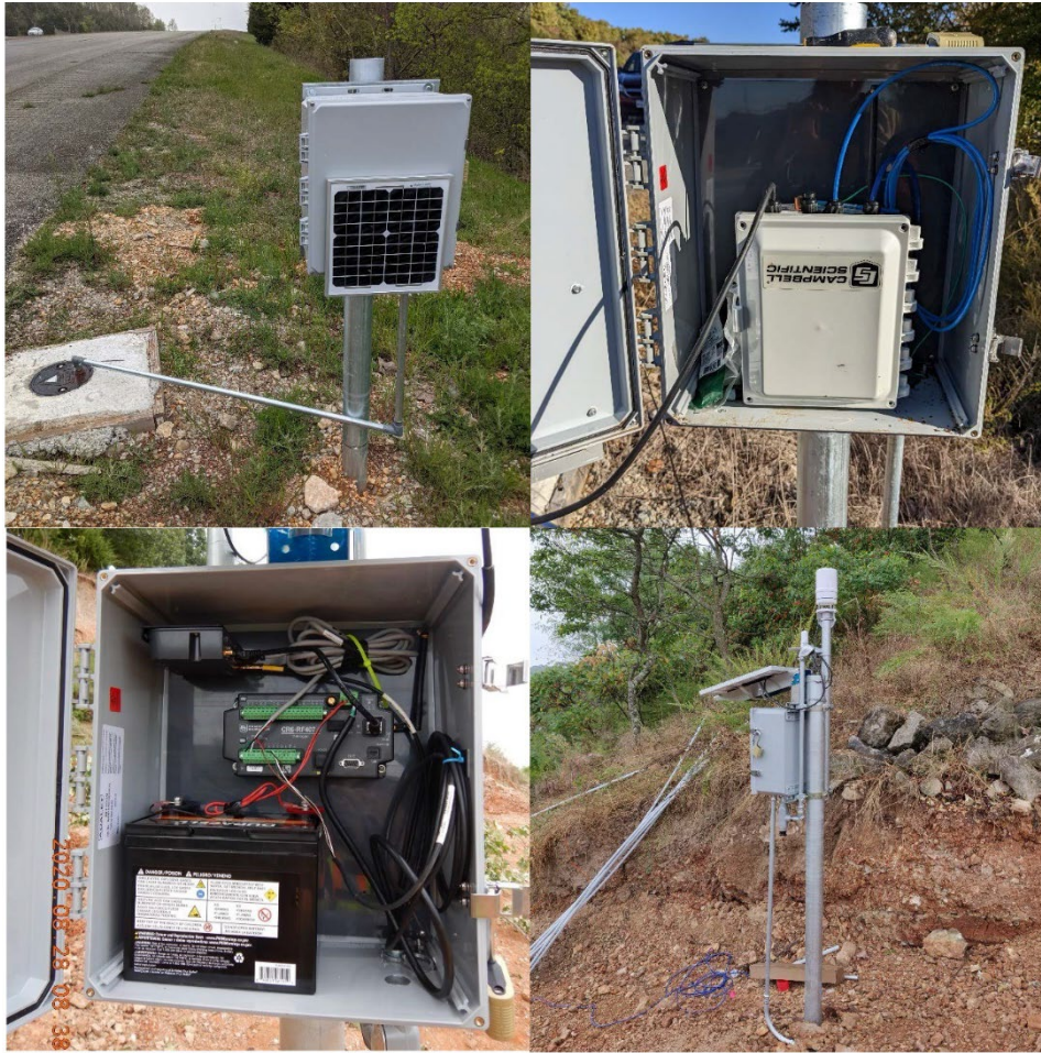
Figure 19: Clockwise from left: weatherproof box and solar panel at LT-3; enclosure with a CRVW3-407 datalogger at LT-3; weather station, solar panel, and weatherproof box at base station; and interior of base station with CR6 logger, peripherals, and rechargeable battery.
