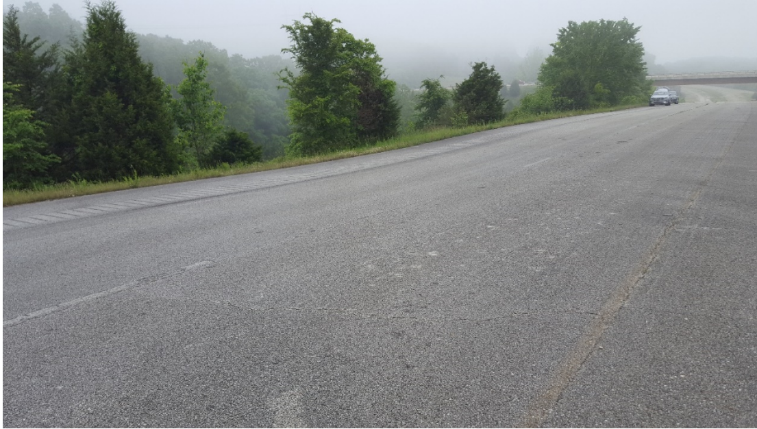
Figure 11: Deformation in shoulder of northbound lanes evidenced by the observed pavement down drop.
