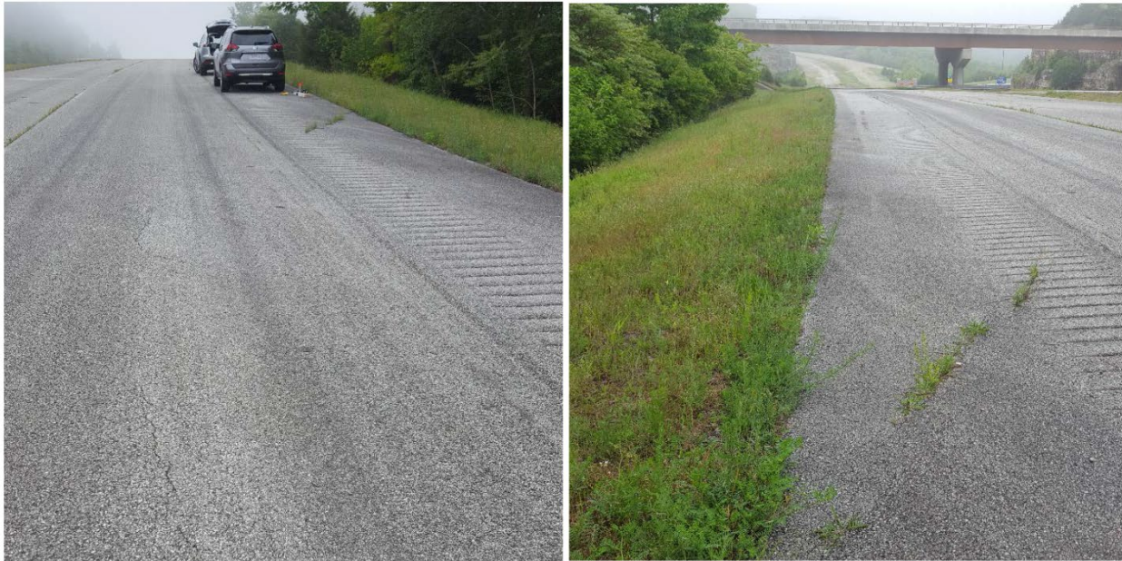
Figure 10: Arcuate cracking and minor deformation of the shoulder in the northbound lanes upslope from the gabion basket retaining wall system.
