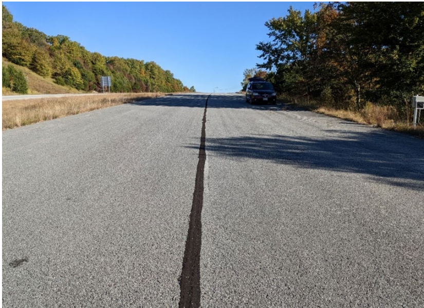
Figure 41: Crack sealing in northbound lane. Photo taken October 2022. LT-3 data logger is visible left of the shoulder.
