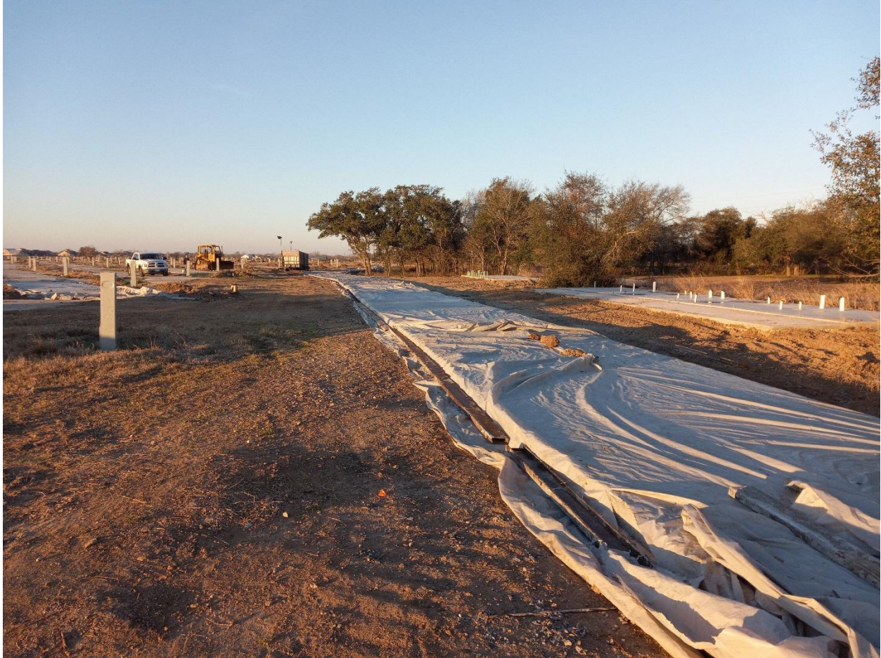
Figure 4-6 A concrete roadway that was cured with Pulp Cure and then covered with plastic.
