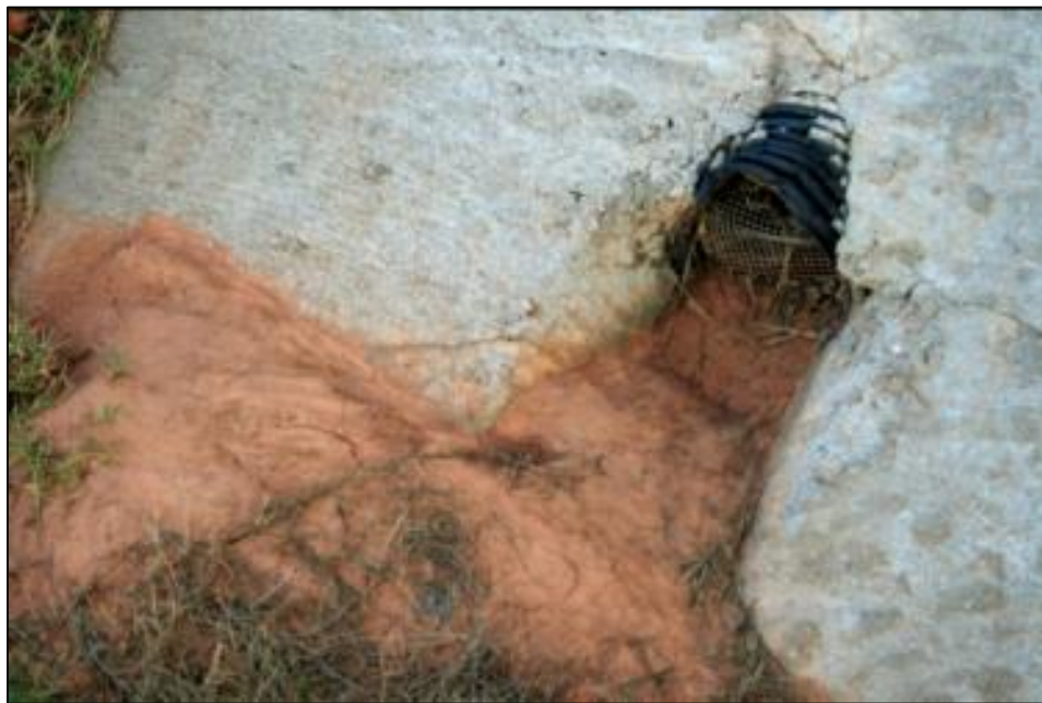
Figure 121. Soil flowing out of underdrain outlet.
