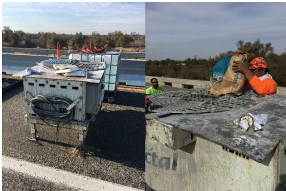
Figure 90. High shear pan mixer in place on the bridge deck (left) and placement of UHPC materials in the mixer (right)
