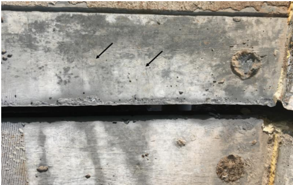
Figure 78. UHPC joint headers on SH-3E bridge before joint sealant was placed and showing hairline cracks
