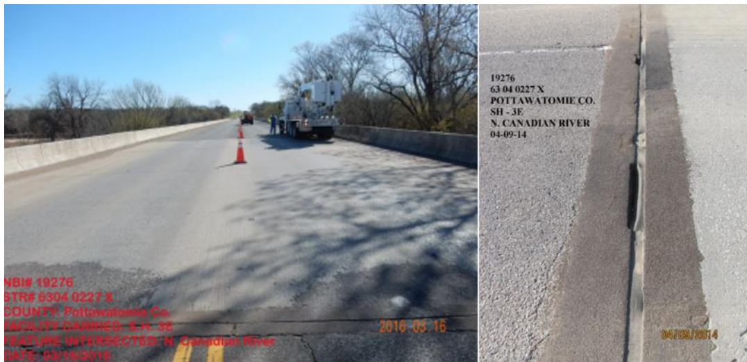
Figure 66. SH-3 bridge over N. Canadian River (left) and expansion joint to be replaced (right)
