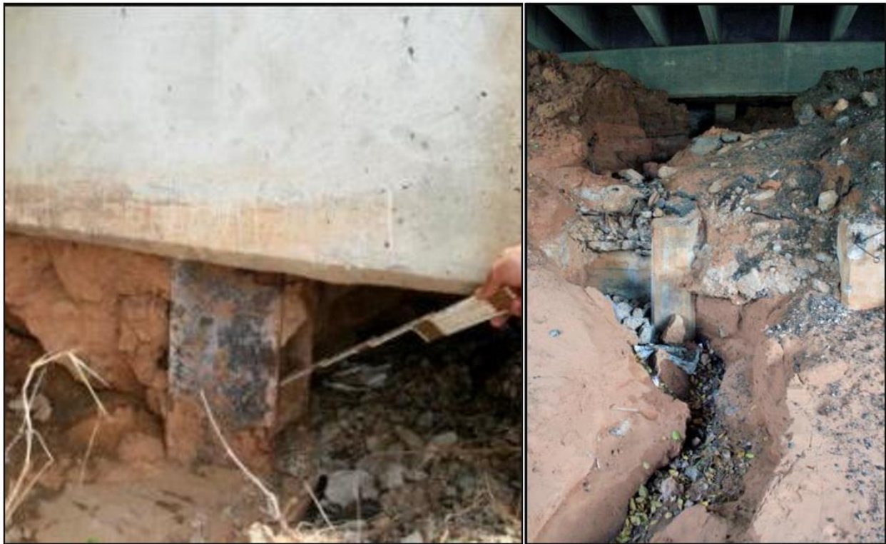
Figure 112. Erosion observed under abutment at Bridge B on US177 over the Salt Fork River (left photo) and at the bridge on SH152 over Willow Creek (right photo)
