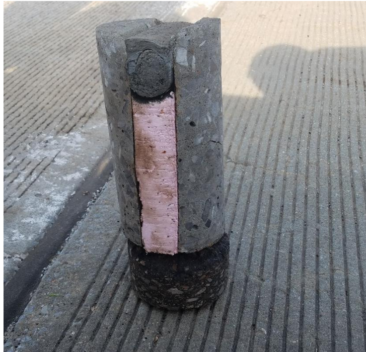
Figure 26. Shields Boulevard over I-40: Expansion joint pavement core
