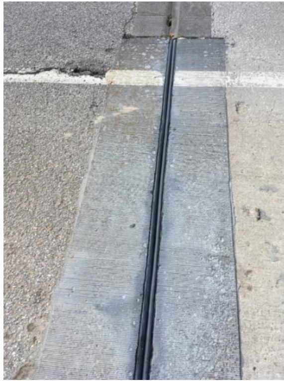
Figure 77. UHPC joint headers on SH-3E bridge immediately after BEJS material was placed
