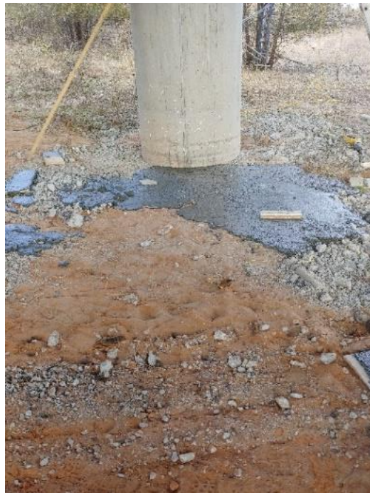
Figure 93. UHPC from failed formwork
