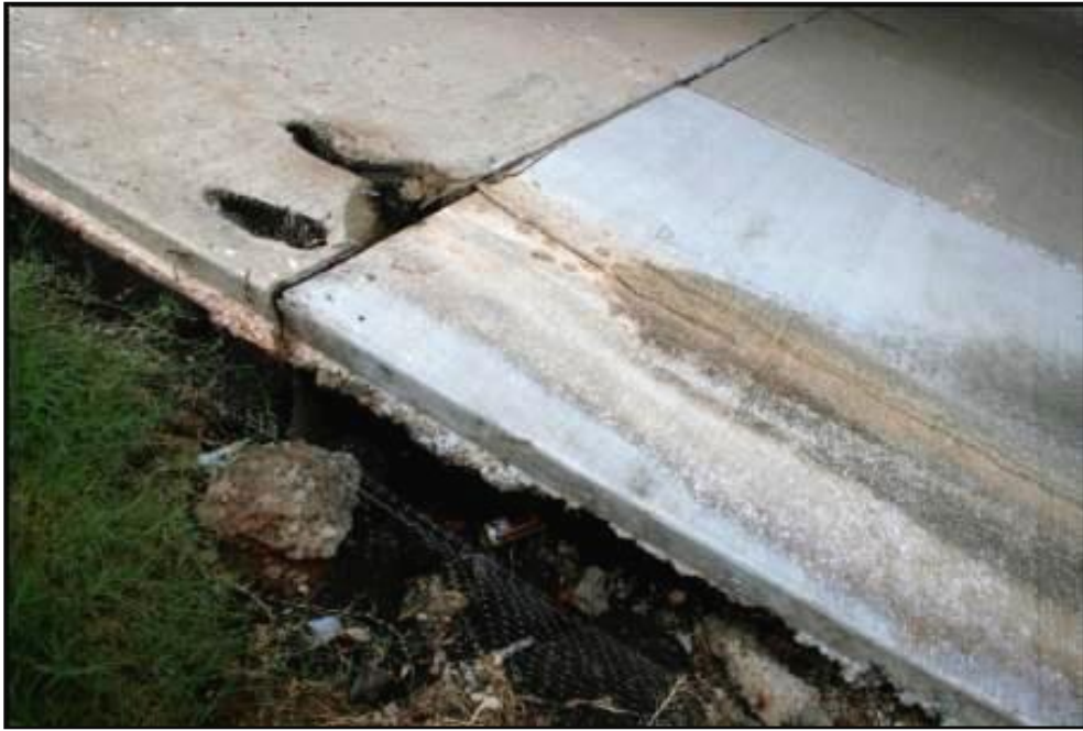
Figure 122. Water flowing from underdrain outlets onto slope wall, Tecumseh Rd. over I-35. (note large void under slope wall)
