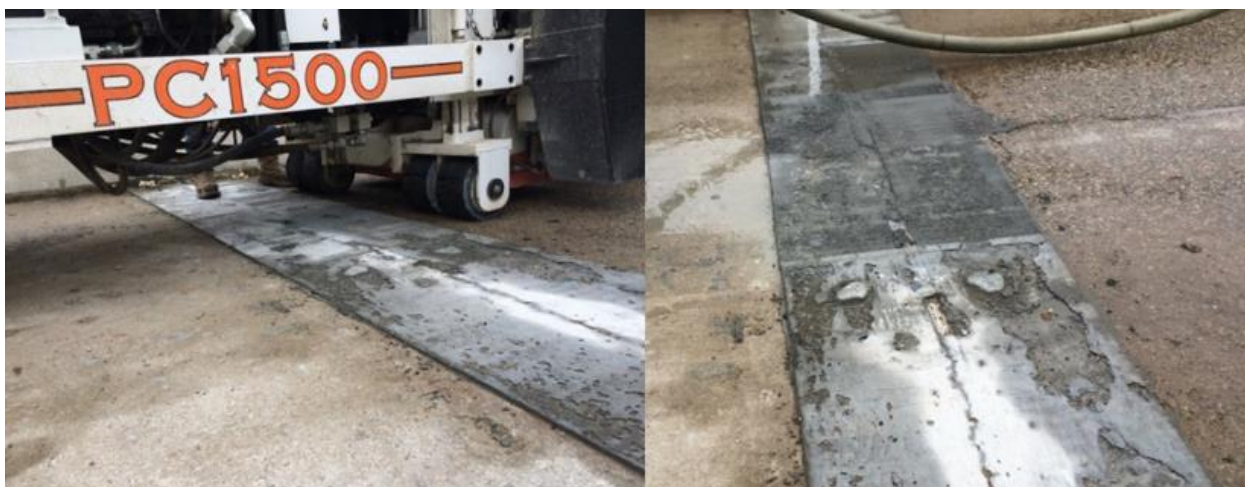
Figure 73. UHPC joint before (left) and after (right) grinding
