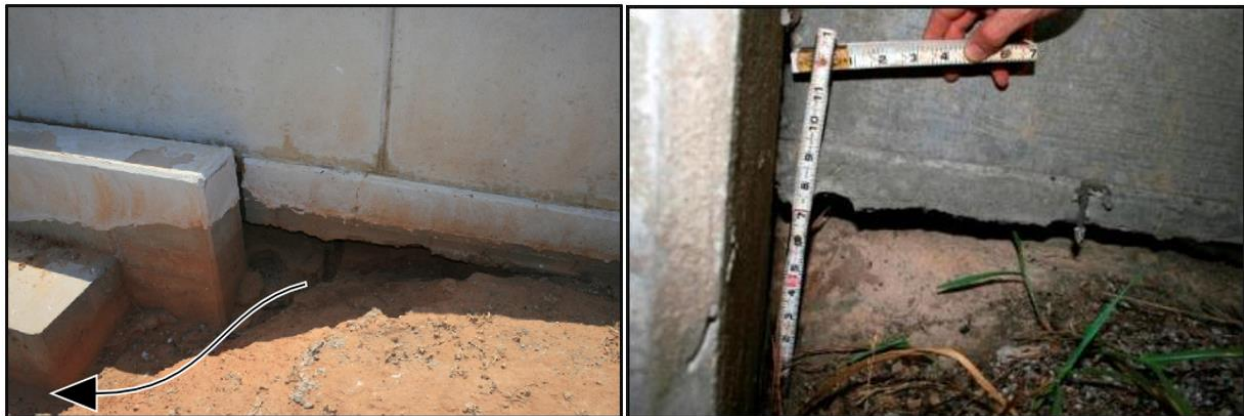
Figure 111. Void beneath approach slab and possible path for water flow (black arrow) at bridge over Sadler Creek (left photo), and another under the approach slab at SH59A over Big Creek (right photo)
