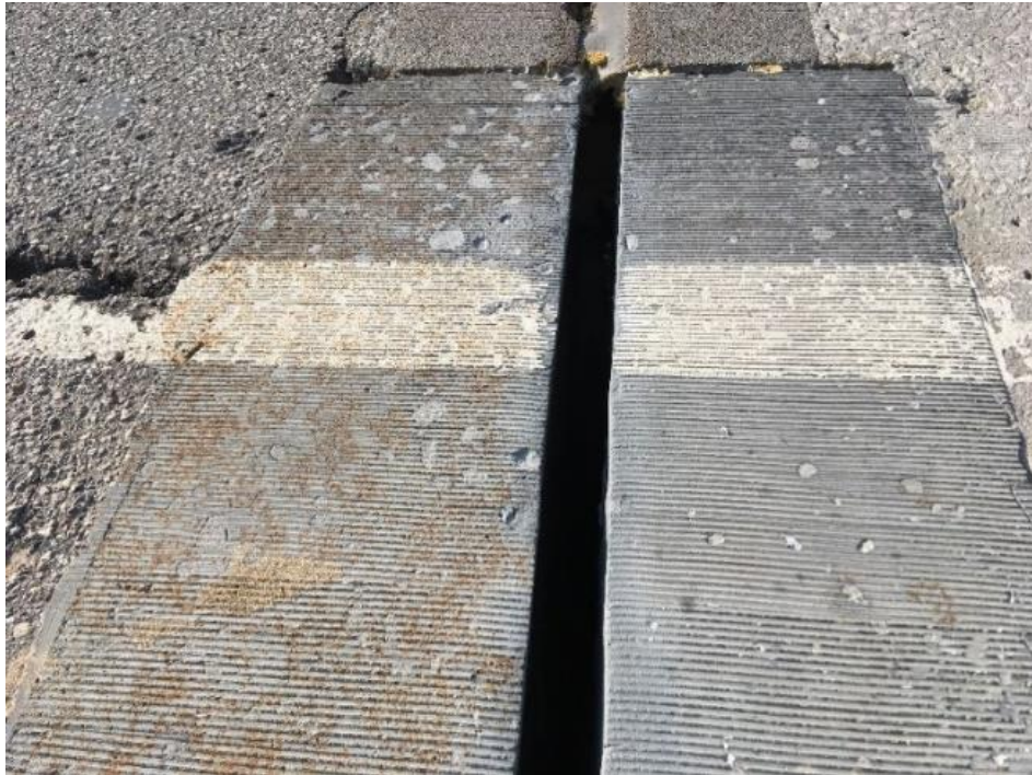
Figure 79. UHPC joint headers on SH-3E bridge before joint sealant was placed and showing surface rusting of the exposed steel fibers
