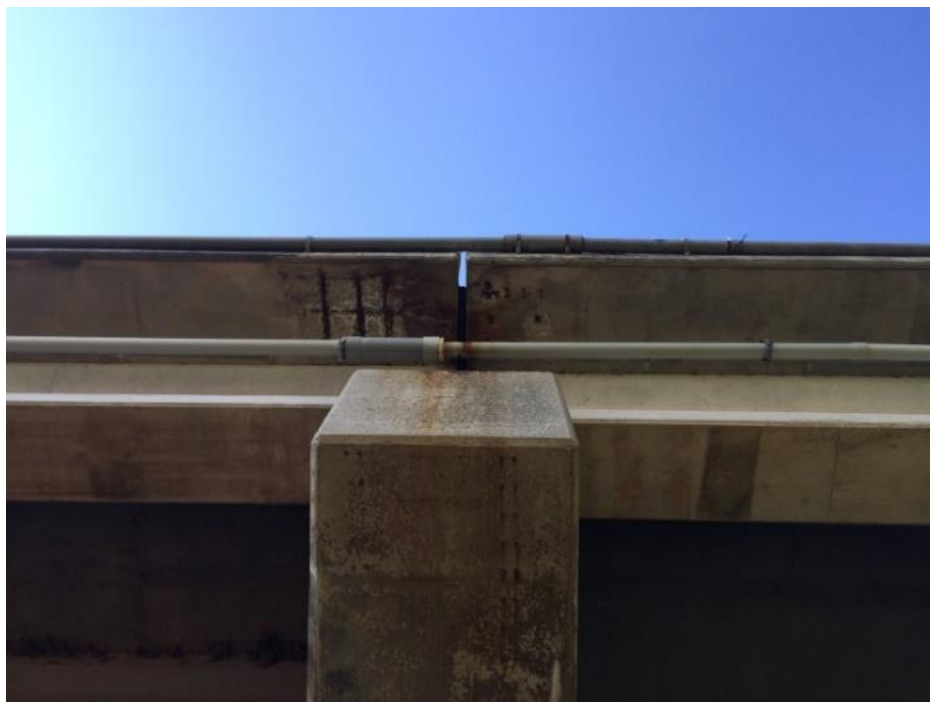
Figure 67. Underside of the SH-3 bridge over N. Canadian River at the candidate joint showing concrete deterioration
