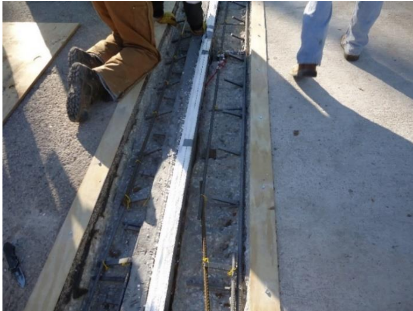
Figure 70. Joint after removal of existing concrete and before placement of the top form
