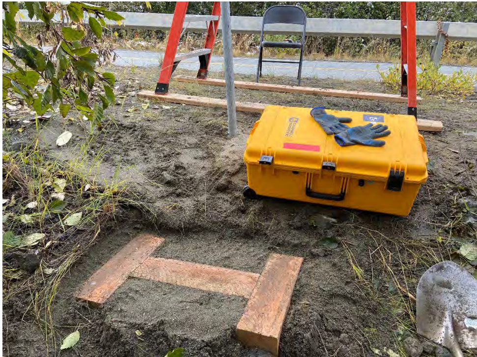
Hatcher Pass MP 15: treated timbers used as solid base for yellow battery box.
