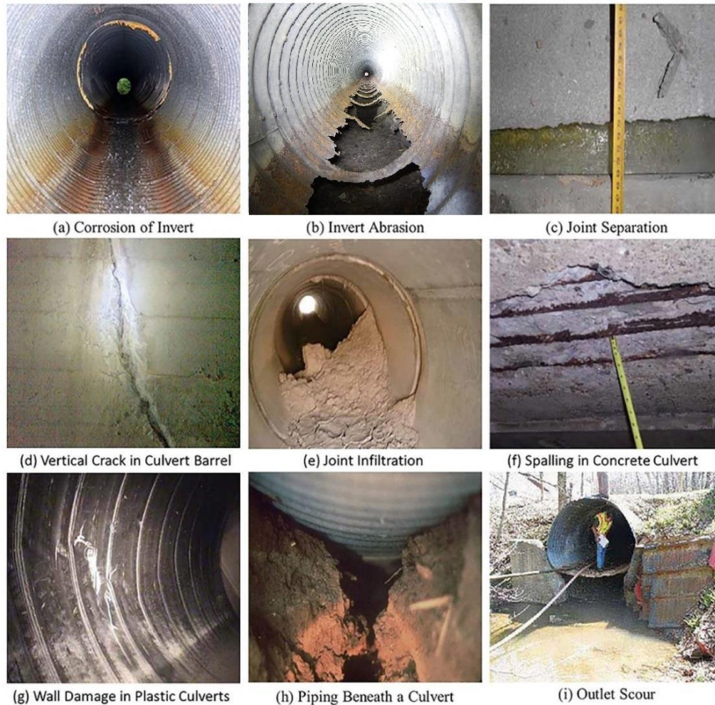
Figure 2- Common culvert defects (Piratla et al., 2019)
