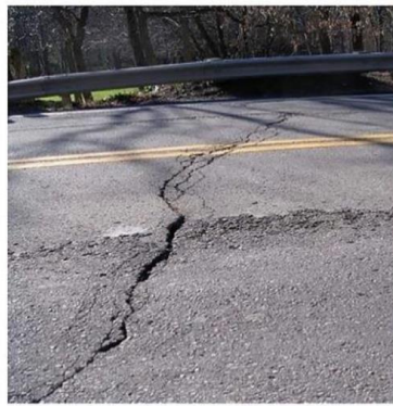
(b) Transverse Crack in the Pavement
