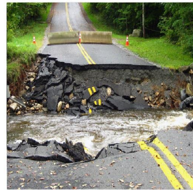
(c) Roadway Collapse Due to Culvert Failure
