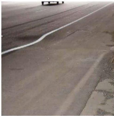
(a) Road Settlement Due to Piping
