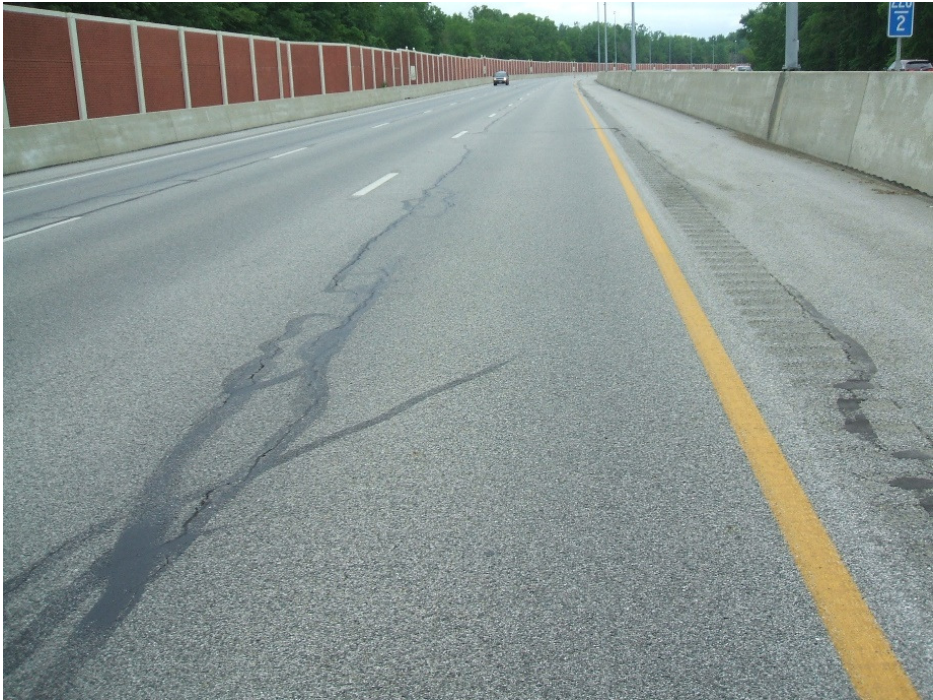
Figure 10. LAK-2 WB lane stabilized section looking east at multiple longitudinal cracks.
