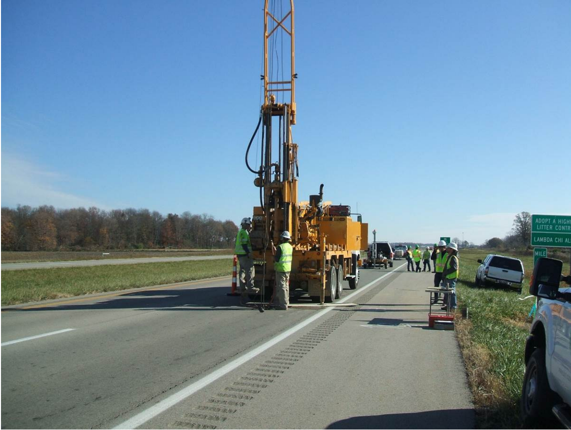
Figure 8. Preparing for SPT testing in foreground, DCP testing and coring in background.
