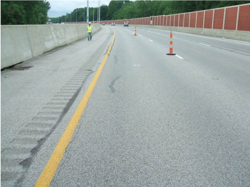
Figure 9. LAK-2 WB lane undercut section looking west at a single longitudinal crack.
