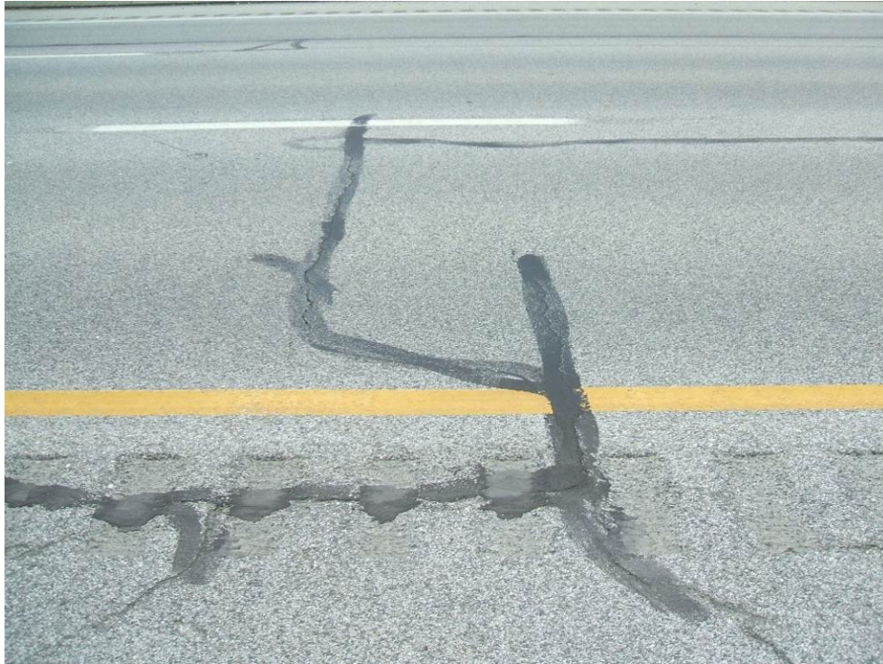
Figure 11. LAK-2 WB lane stabilized section looking north at transverse crack.
