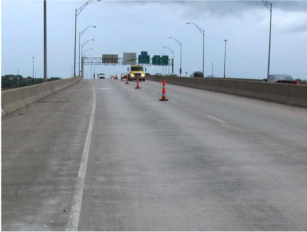
Figure 3.13. Deck surface showing surface texture and color variation between wheelpaths and surrounding deck.
