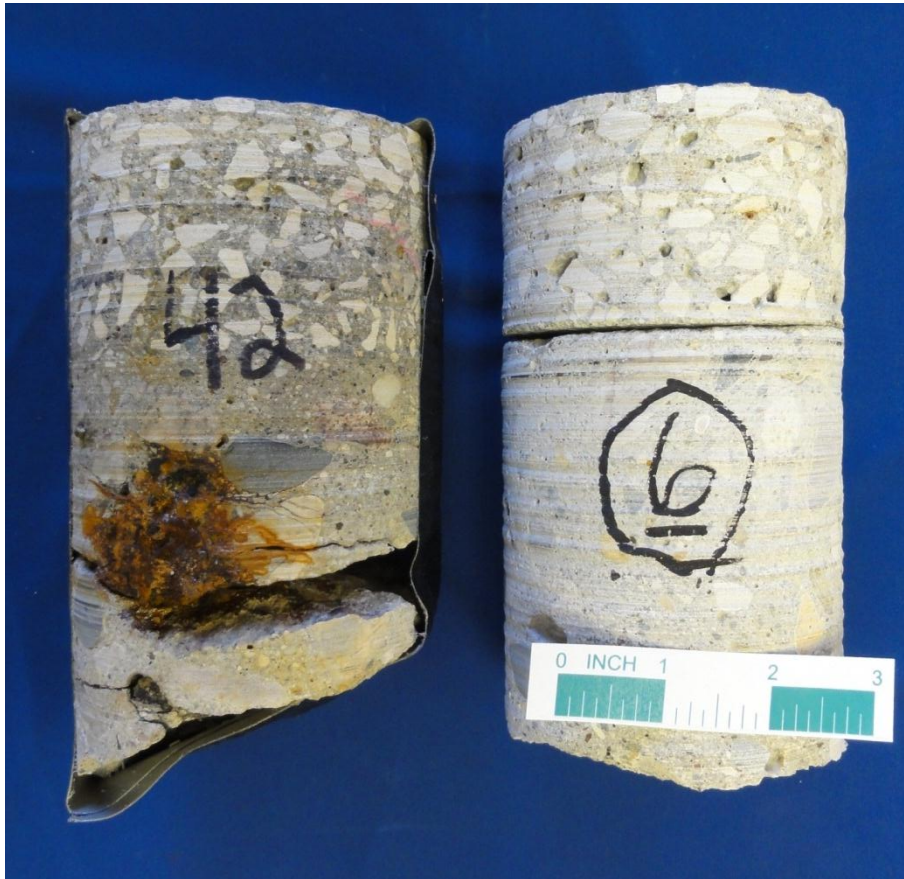
Figure 1. Core 6 and 42 as received for petrographic studies. Topping layer in Core 6 as received was delaminated from the base concrete.
