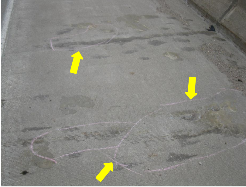
Figure 2.10. Delamination in shoulder (highlighted in chalk). Note epoxy injection resin on the surface.
