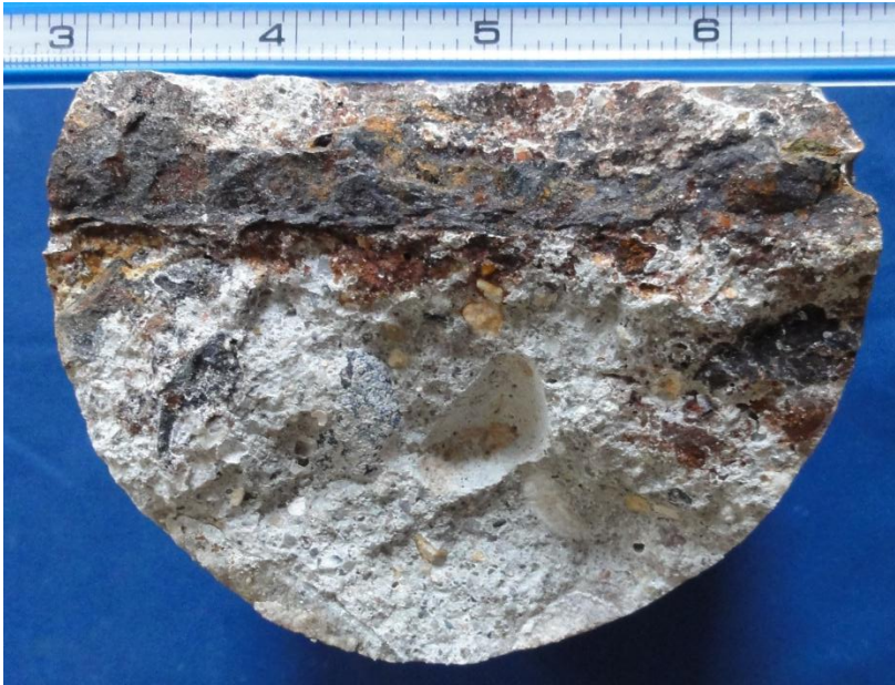
Figure 8. Core 42; corroded rebar in base concrete at one of the transverse cracks.
