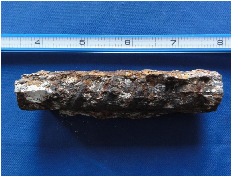
Figure 9. Core 42: corroded rebar taken out of base concrete at one of the cracks.
