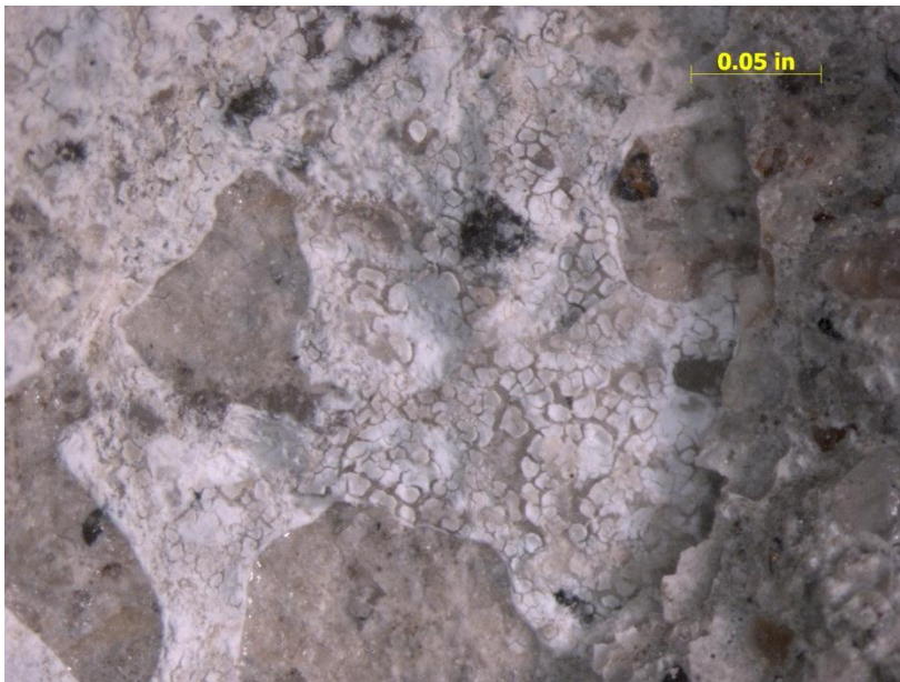
Figure 11. Core 42; close up of the light color area of the bottom surface of the core from Figure 8 showing that the surface is coated with ASR gel.
