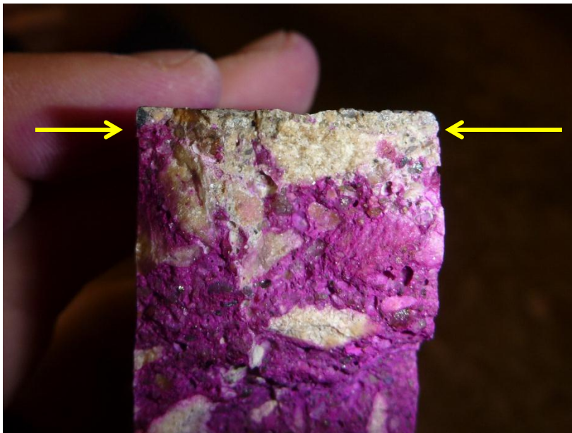
Figure 8.2. Phenolphthalein indicator on a freshly cracked surface of a core. The depth of carbonation is indicated by the arrow (pink color indicates pH > 9 ).
