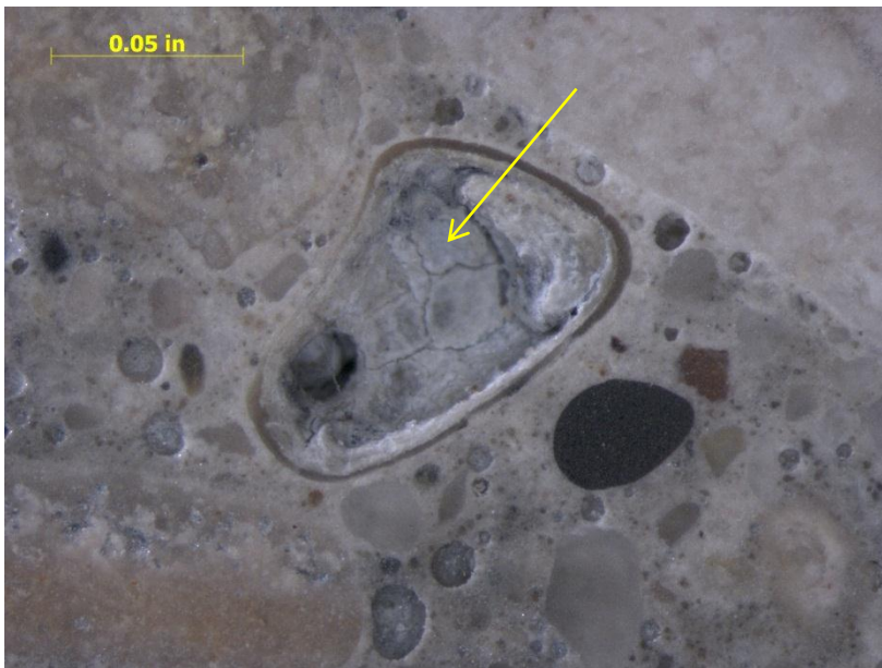
Figure 5. Core 6 topping; the largest reacted fine particle of shale (encircled in Figure 2) located in close proximity to the intercepting microcracks. Most of the interior of this particle has been consumed in the alkali-silica reaction; gel was found on the surfaces of the microcracks.
