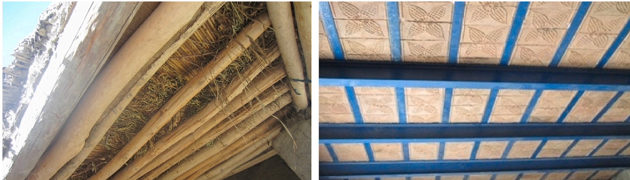
Fig. 3. Bamboo mat roof, using wooden poles (Left), Ceiling construction using bricks and I/T-beams (Right).
