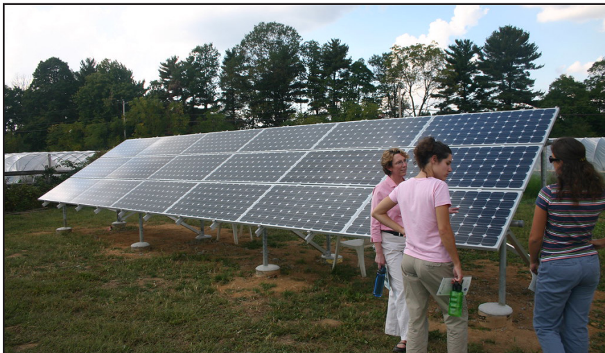
Figure 1.13: Demonstration solar panel at the Pennypack CSA, Montgomery County, MD. Source: Pennypack CSA, Montgomery County, MD
