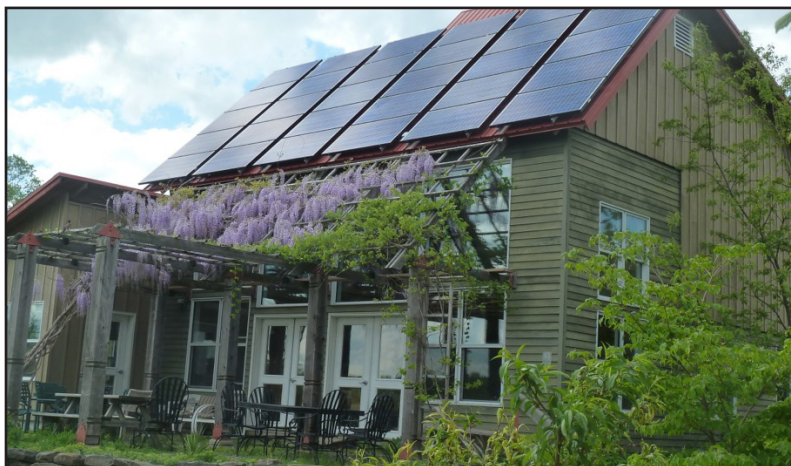
Figure 4.37: Rooftop Solar. Source: EcoVillage at Ithaca, n.d.
