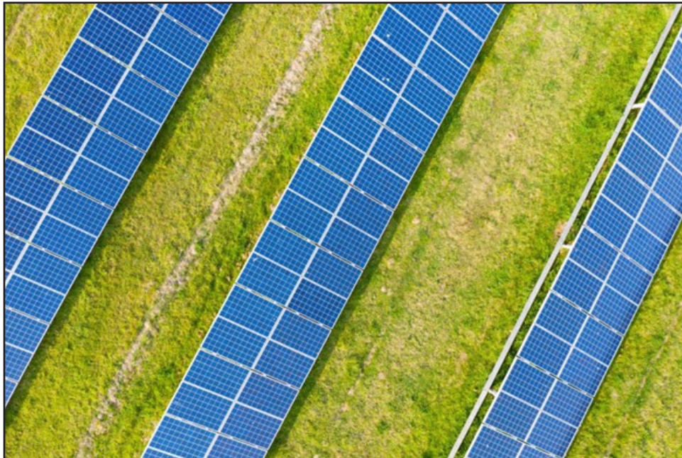
Figure 4.22: Ground-mounted solar panel project from above.
