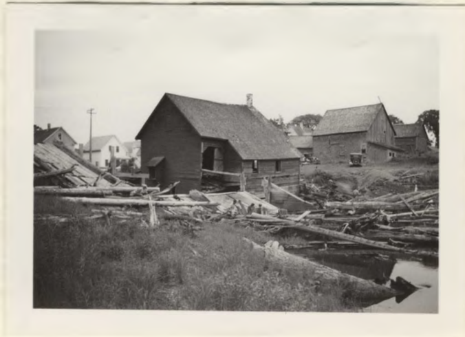
This scene represents the activities of the crews to rebuild the old Jewett-Durrell grist mill. See page 110.
