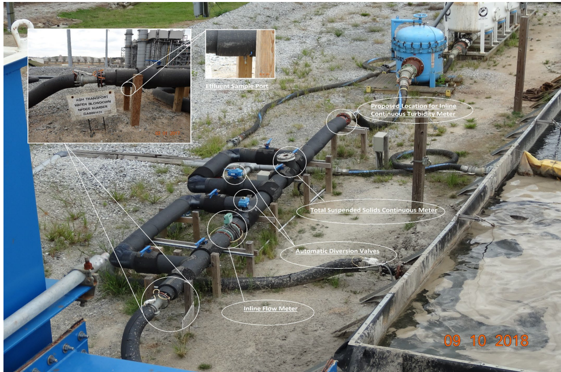
Phys-Chem WW Treatment Package Plant
