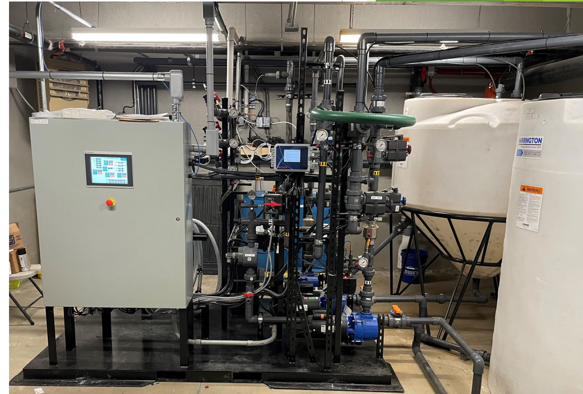
Hoganas - Clean-IT Treatment Package Plant
