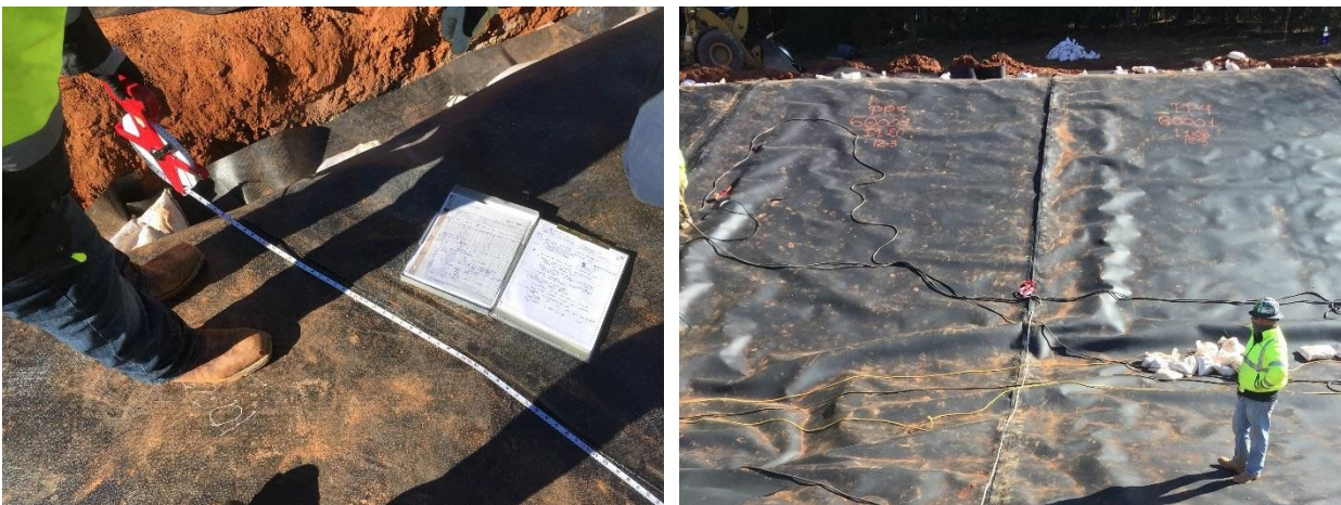
Figure 10: Top shows graphical pressure report of out of tolerance pressure readings with CQA location descriptions and explanations. Photo on the bottom left shows a typical anchor trench location recorded with low pressure; photo on the bottom right shows the location of a wrinkle that recorded low pressure.
