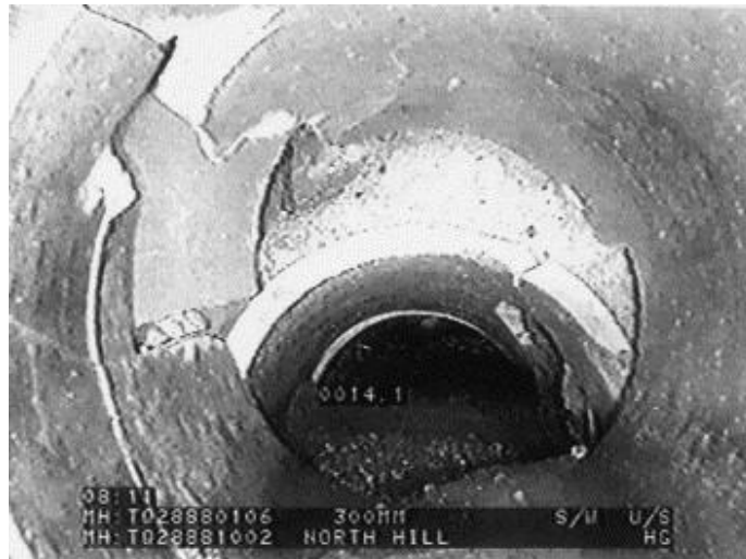
Figure B46. Cracked sewage pipe.
