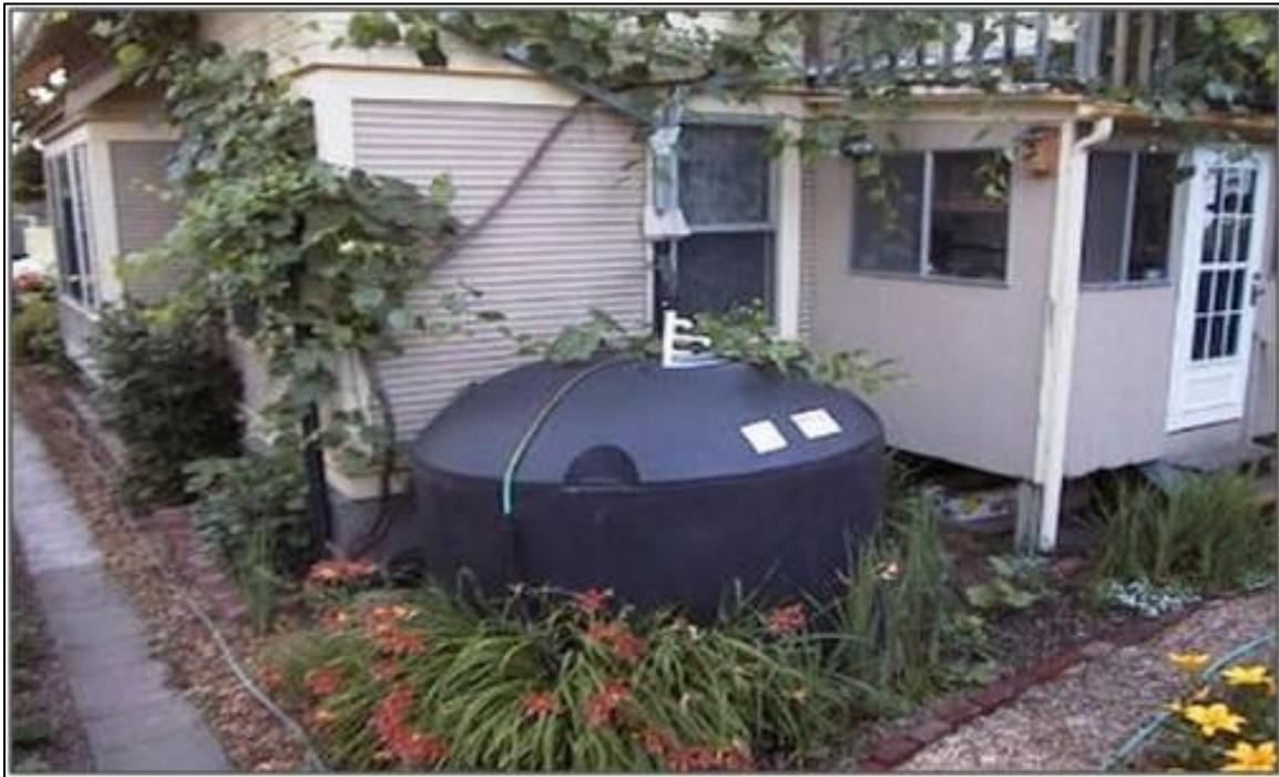
Figure B40. Household cistern for collecting rainwater.
