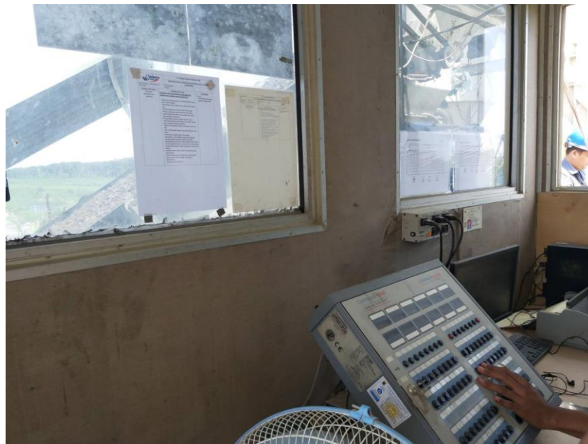
Gambar 2.1 Control Cabin Unit Batching Plant Waskita Beton Precast
