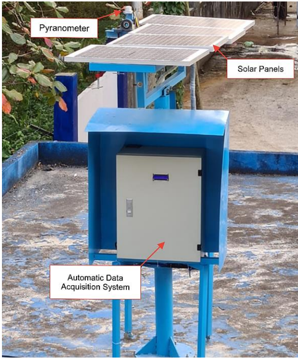
Figure 3. Installed low-cost PV monitoring system.
