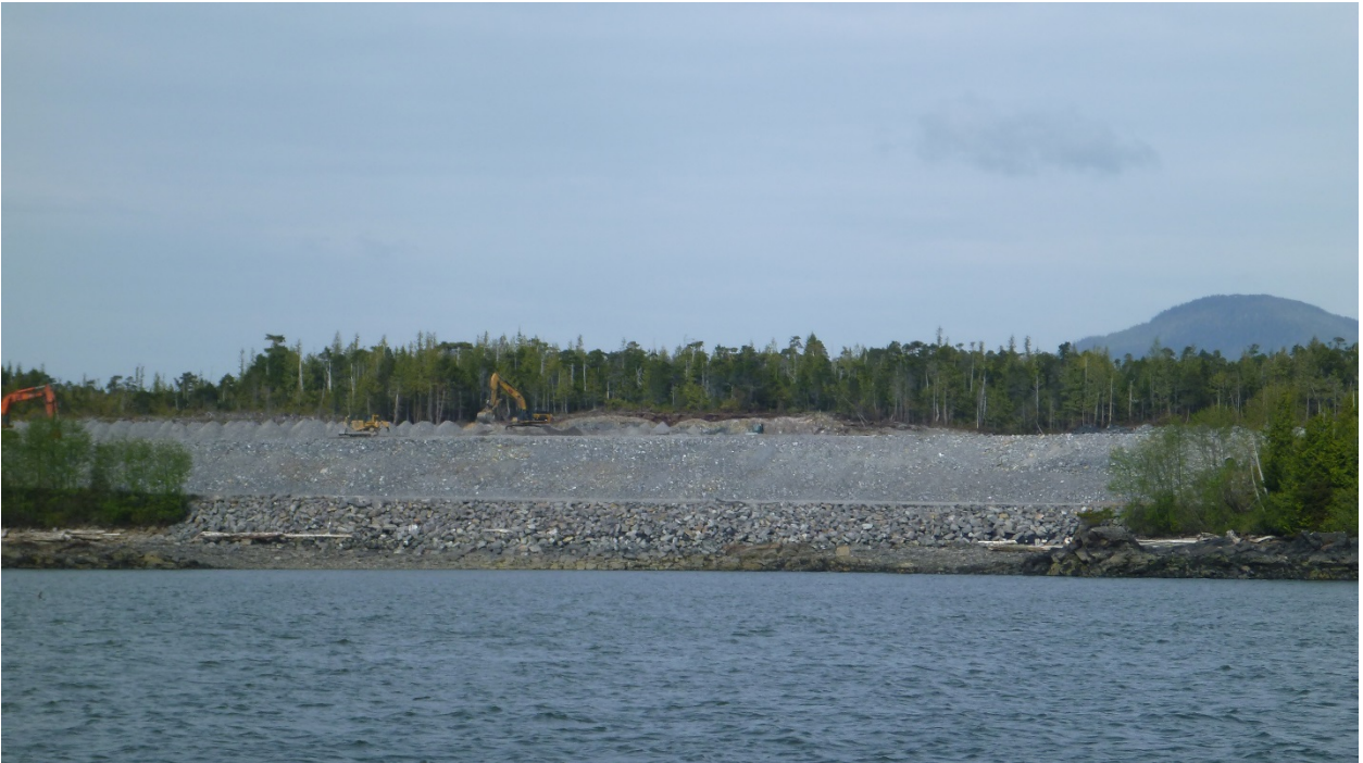
Figure 4.1. Foreshore modifications including shoreline armoring and removal of riparian habitat on Ridley Island during construction of a road, rail and utility corridor.
