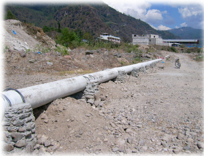
Image 6. Tubing installed by community group through private and public land to redirect waste-water through new and pre-existing wetlands 28
