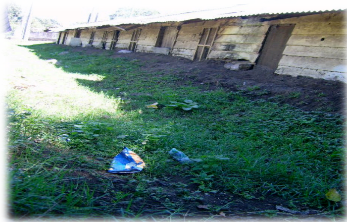
Image 7. Previous sediment build-up blocking entrances to building in the town of San Lucas 47
